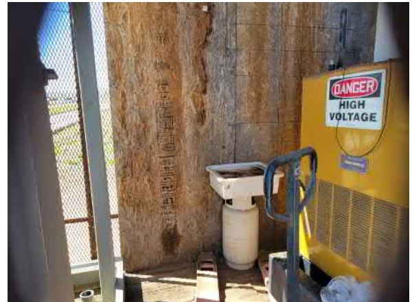
Photo #8 View of generator, located on the north-central portion of the site.
