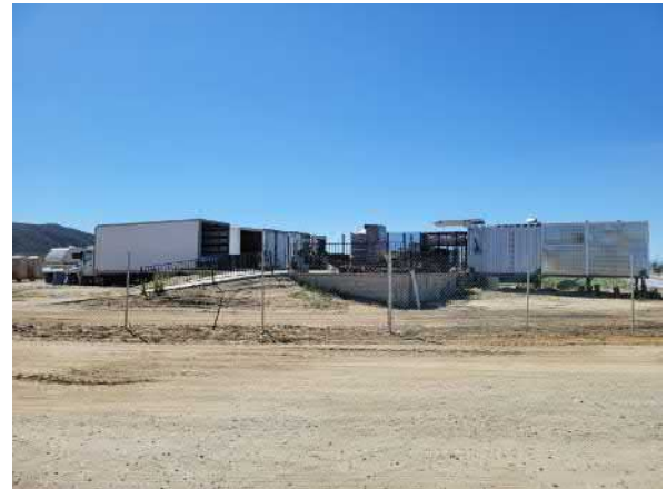
Photo #4 View of on-site trailers, located on the north-central portion of the site.
