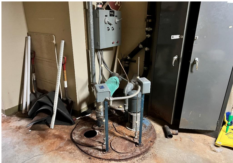
Photograph 6: View of sump pump located in the basement beneath the eastern portion of the property.
