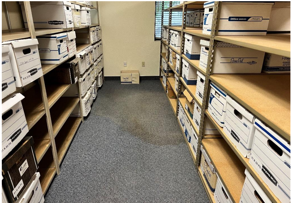
Photograph 4: View of water stains on the carpet in the file room at the eastern portion of the building.
