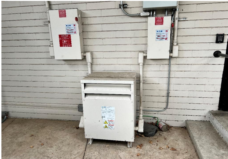
Photograph 2: View of transformer located at the southeastern portion of the building.
