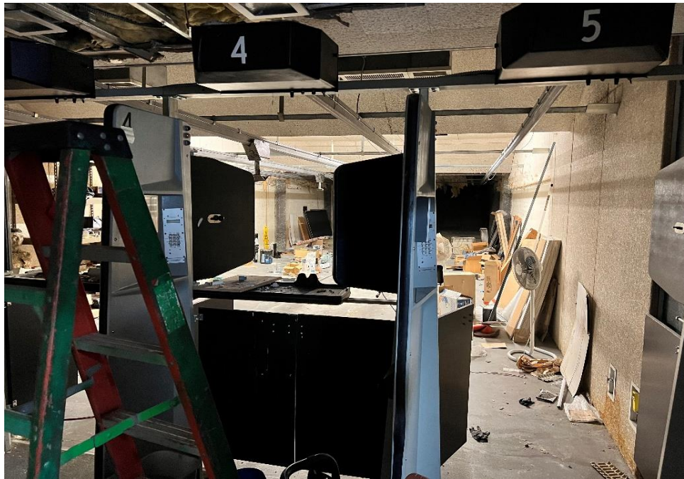
Photograph 7: View of shooting range in the basement beneath the eastern portion of the property.
