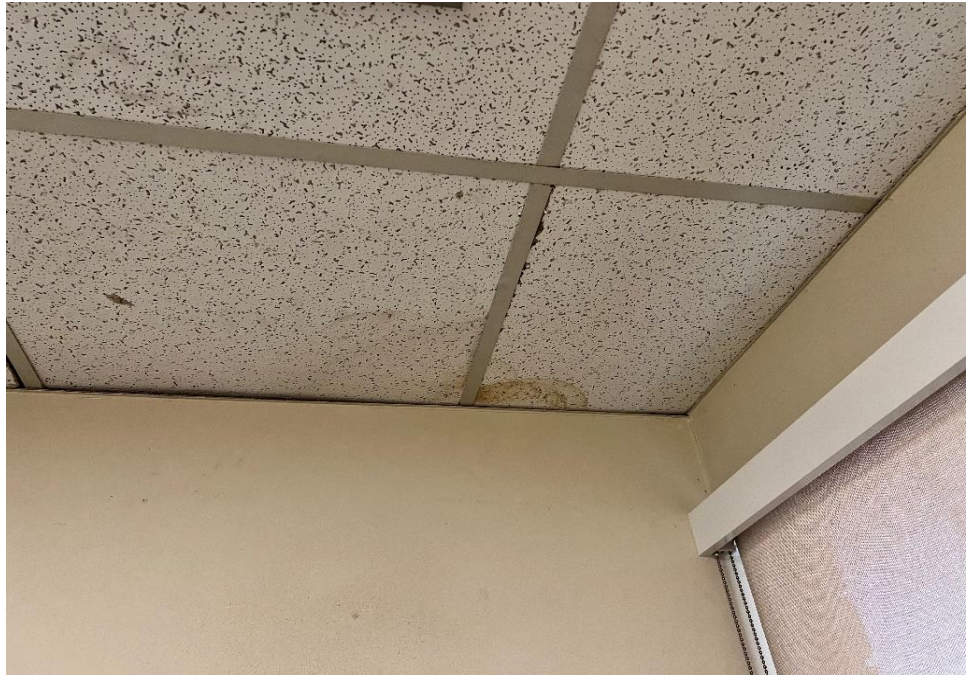
Photograph 3: View of water stain on ceiling panels located at the southeastern portion of the building.
