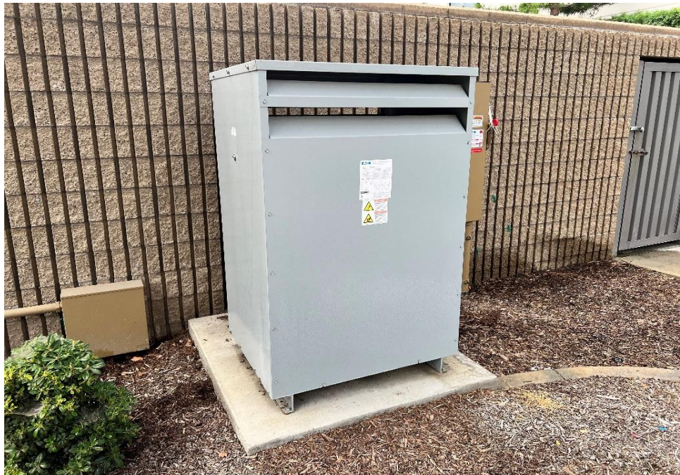
Photograph 14: View of transformer located at the southwestern vicinity of the site.
