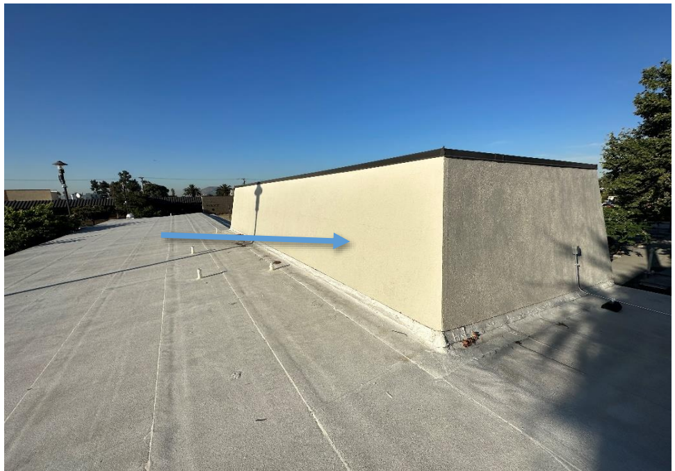
Photograph 2: Representative view of the exterior stucco associated with the asbestos containing barrier paper located throughout the exterior walls of the building.
