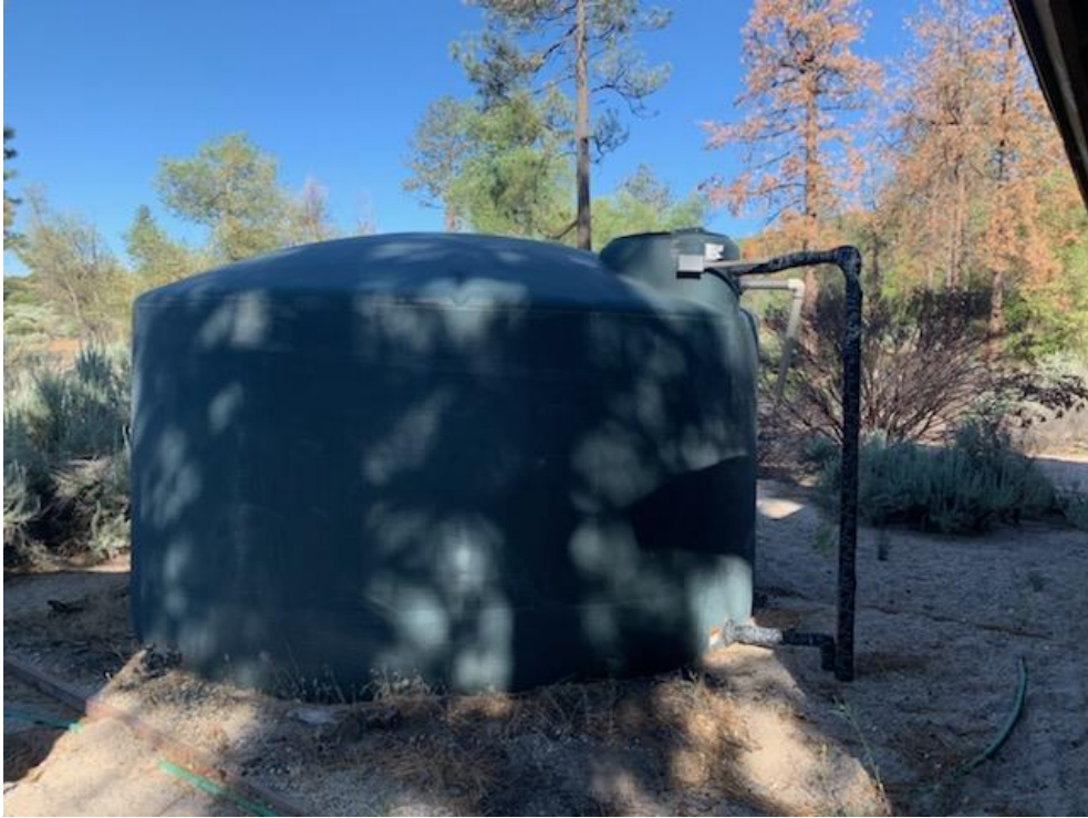
3. View of aboveground water storage tank on the northwest portion of the property.
