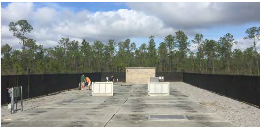
30,000 gallon decentralized treatment system
