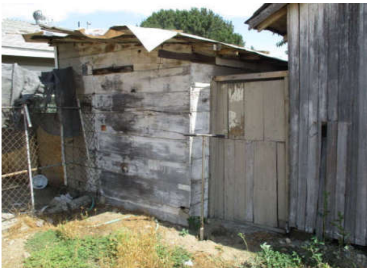
Photo #27: Another view of soil sampling location 6-3 (next to smaller storage shed corner and septic tank [foreground]), looking southeast towards residence at 9092 Catawba Avenue
