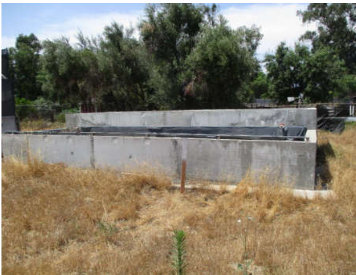
Photo #18: Another view of soil sampling location 5-2 next to concrete fluid storage tubs (2), looking northwest
