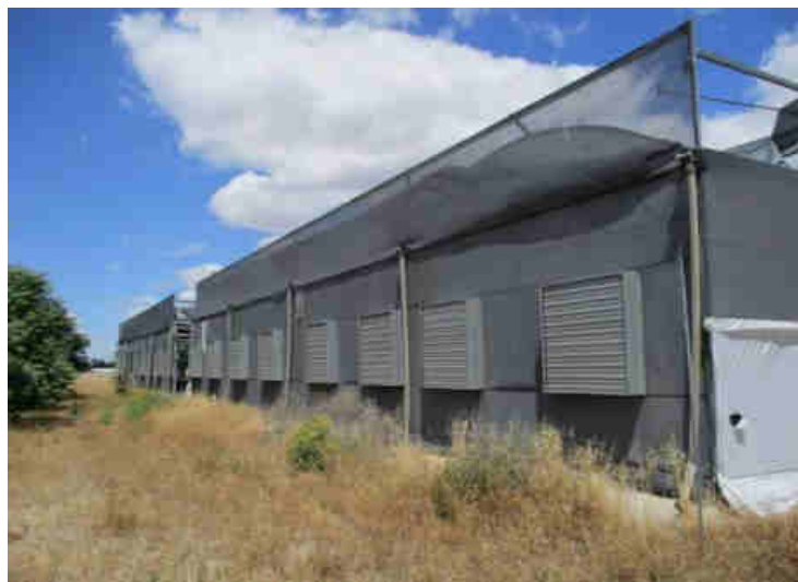
Photo #23: View of two abandoned greenhouses located onsite, looking west
