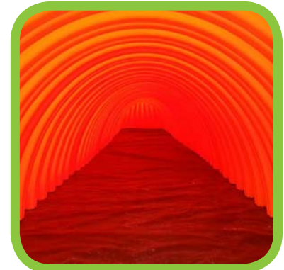
Looking down the Isolator Row from the manhole opening, woven geotextile base between the chamber and stone base.
