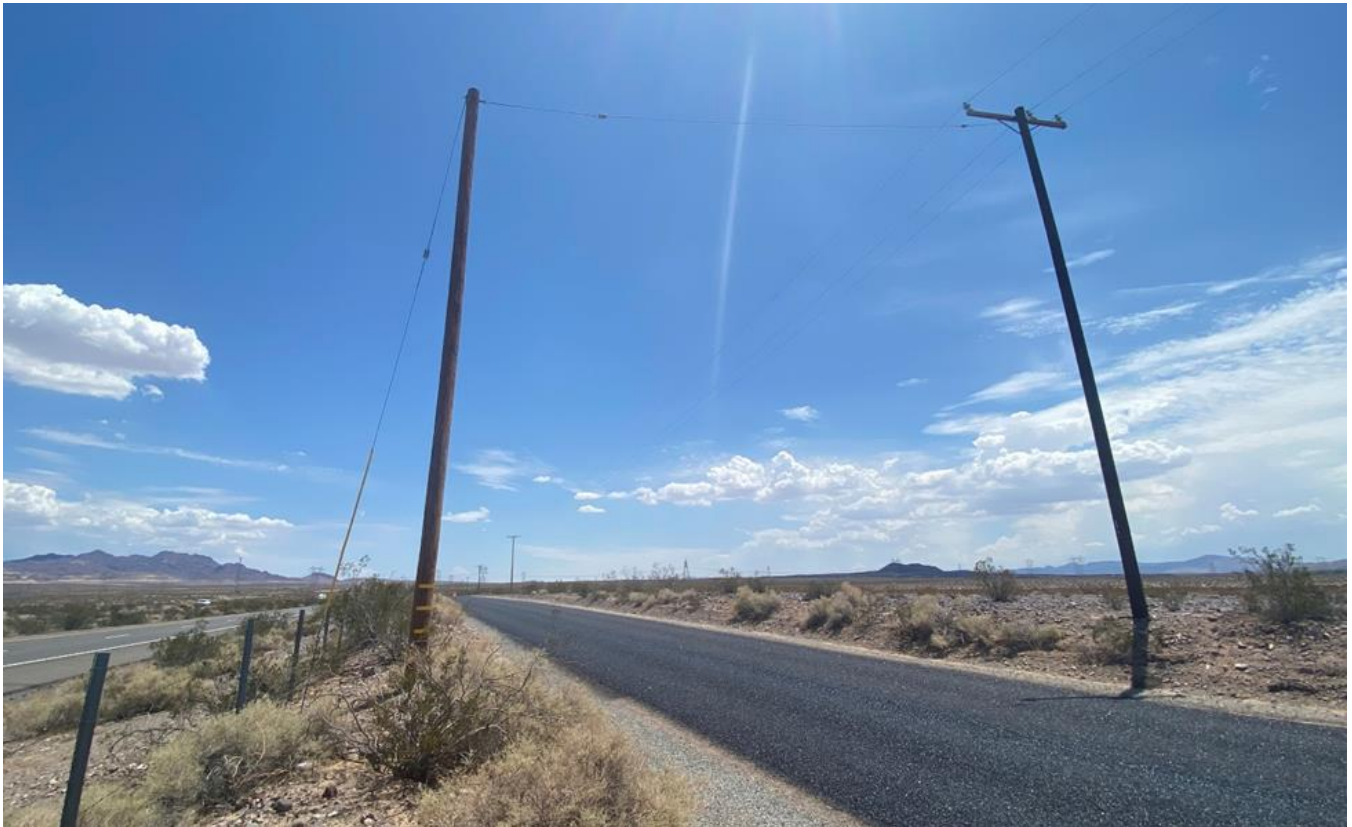
Figure 2. Segment 1 Existing Hector 12 kV/Baroid 66 kV Distribution Line
