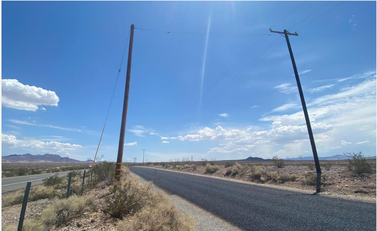
Figure 2. Segment 1 Existing Hector 12 kV/Baroid 66 kV Distribution Line
