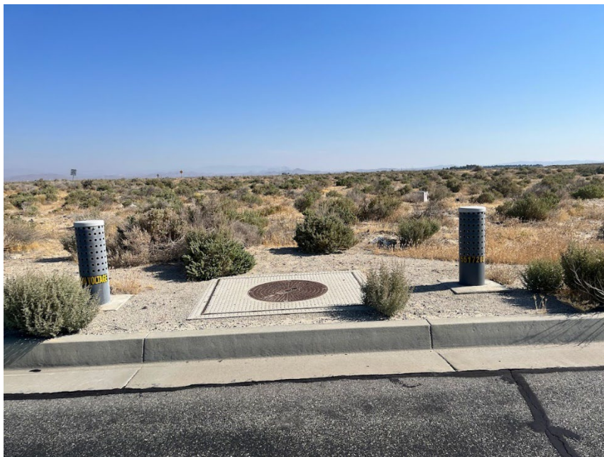
G-8. Southwest Subject Property – Utilities at corner of S 30 th Street West and Avenue G (06/14/2023).
