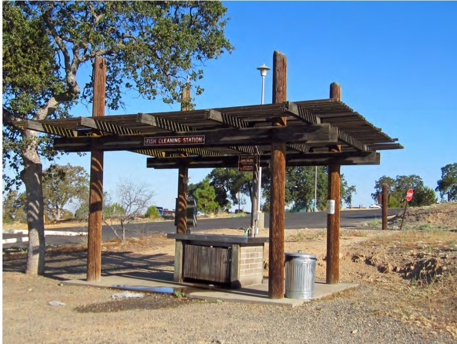
HDR-14a Blue Oaks Recreation Area Fish Cleaning Station, south elevation and east primary façade, View northwest, Photo taken 07/13/12
