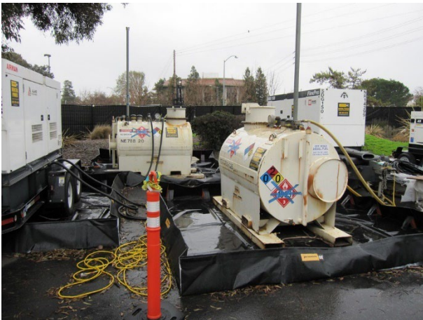
Photograph 3. On-Site generators and ASTs.
