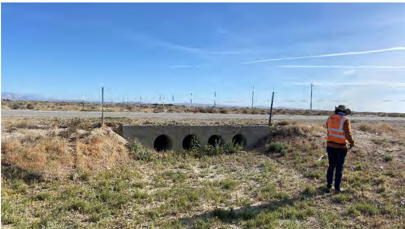
Photograph 3. View of a culvert along the northern boundary of the subject property, facing north.
