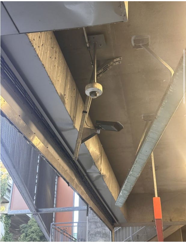
Figure 2: Automatic License Plate Reader Installed
