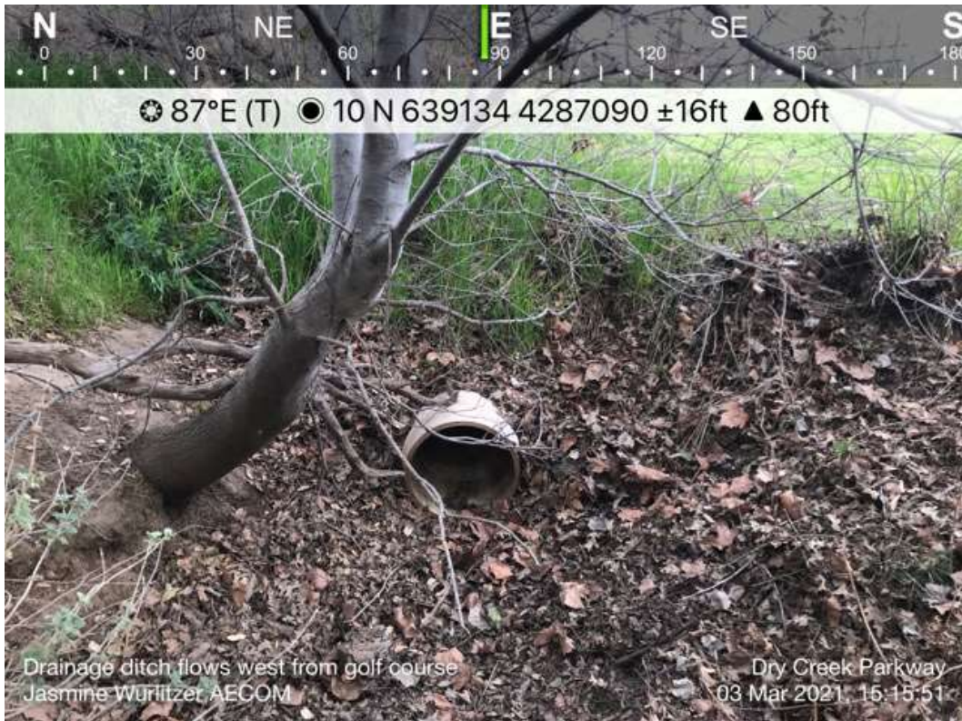
Photo 7. Aquatic Feature Ditch 2 – small ditch with culvert that conveys runoff from Antelope Greens Golf Course to the west.
