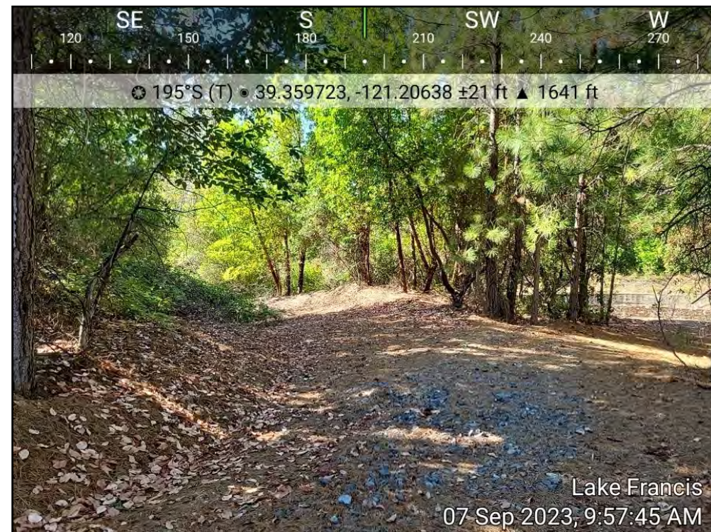
Photo Point 3. View of spillway access road. Spillway wall can be seen on the right side of photo.
