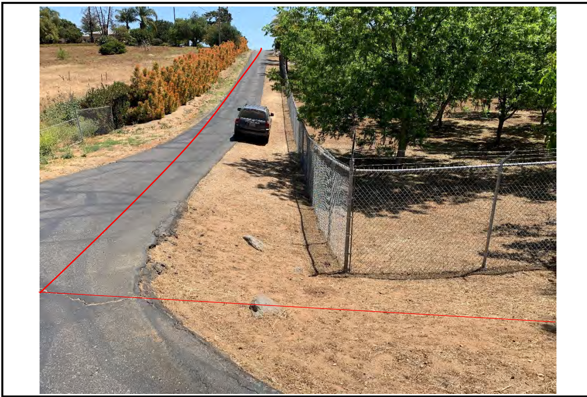
Photo Point 4a. Photo taken at the northern limit of alignment. Red line represents the approximate location of the alignment within view. A culvert is located under the road at this location (north-south). Photo date: 05/05/22. Direction: east. Lat/Long: 33.254244, -117.219581
