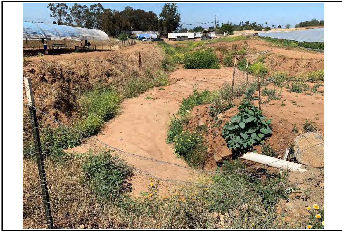
Photo Point 10. Photo of basin. Culverts from the agricultural operation drain into this basin. Basin fills up and drains offsite. Photo date: 05/05/22. Direction: west. Lat/Long: 33.242972, -117.224306
