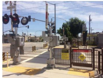
Safety elements of a gate and pedestrian arms have been constructed at the Monrovia Station.
