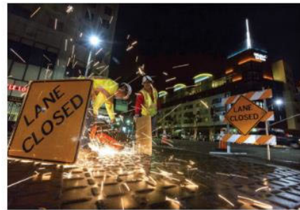
Construction during approved hours ensures the steady progress of adjacent development construction and minimizes impacts to Metro's transit service.
