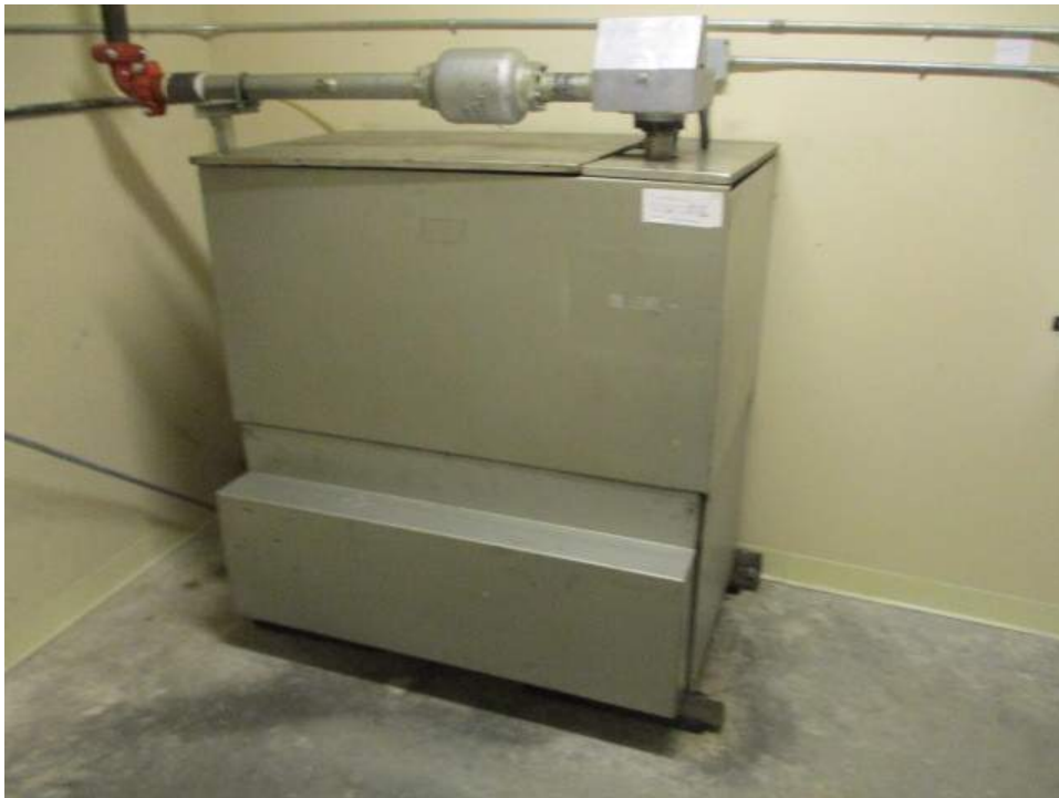
18. Hydraulic elevator unit #2
