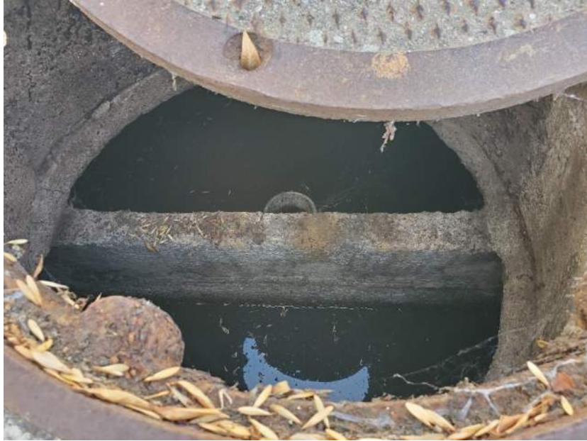
Photograph 11 – Grease interceptor on the north side of the building.
