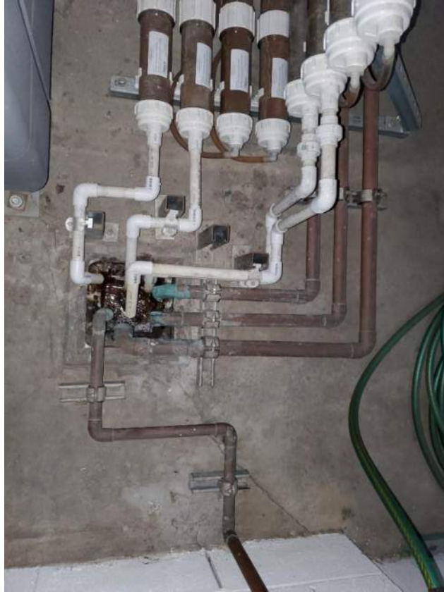
Photograph 29 – Floor drain within first floor mechanical room with piping from condenser units
