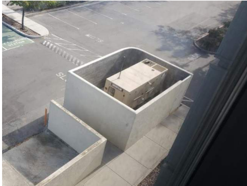
Photograph 7 – Backup generator with 400-gallon diesel aboveground storage tank (AST) on the northeastern side of the building from above.
