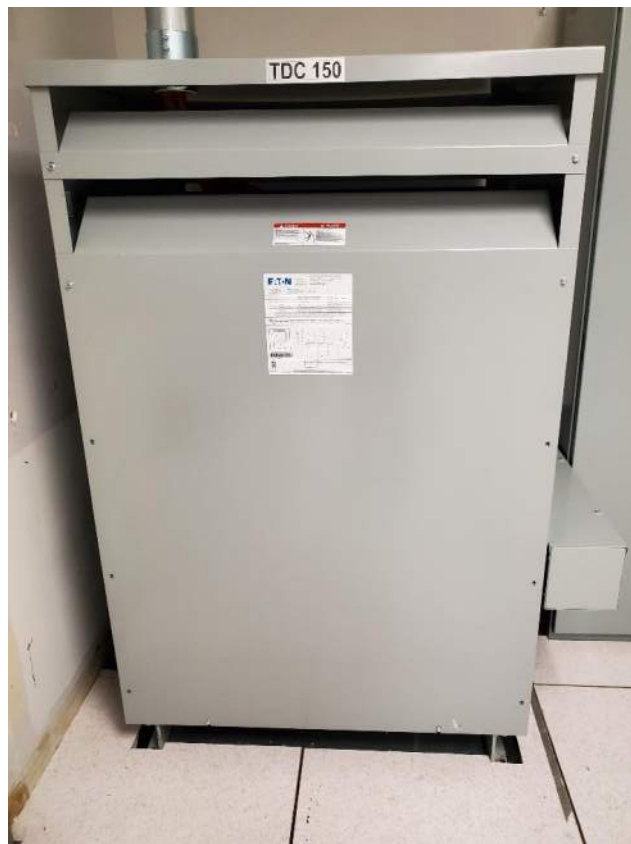
Photograph 32 – Dry transformer within building
