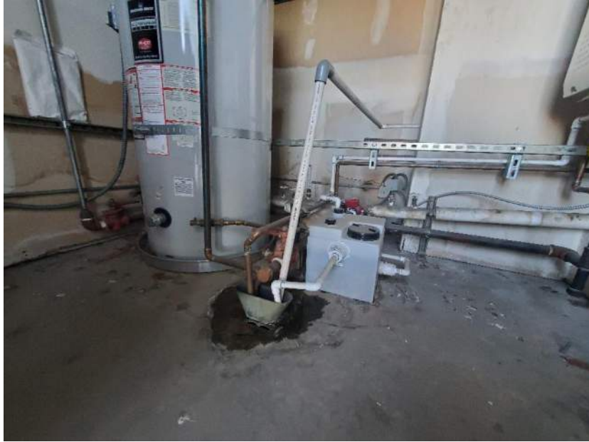
Photograph 17 – Hot water heater within roof mechanical room, facing west.
