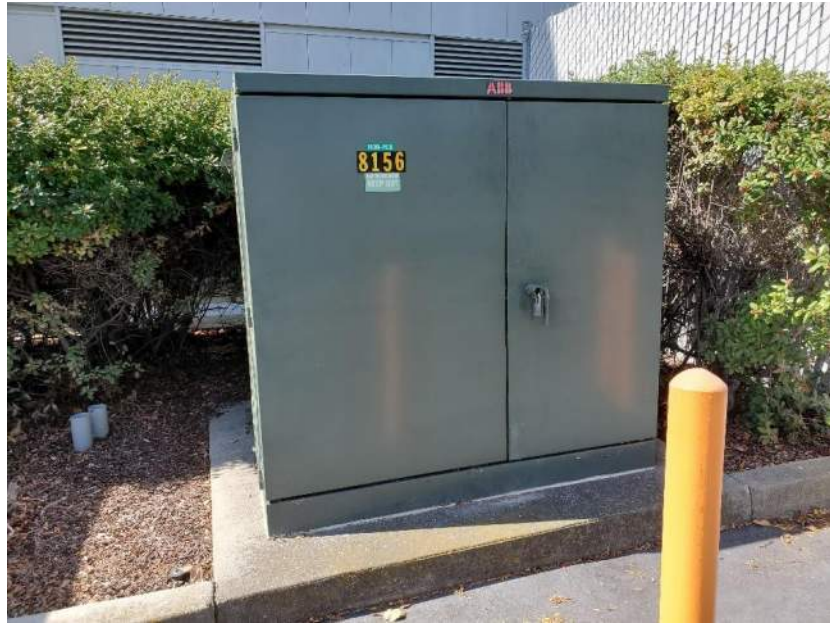
Photograph 15 – Pad mounted transformer on northern side of the building, facing south.
