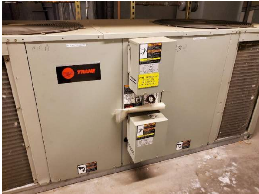
Photograph 27 – First floor mechanical room
