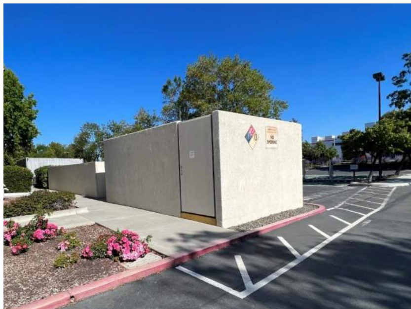
Photograph 8 – Enclosure around AST on the northeastern side of the building, facing west.
