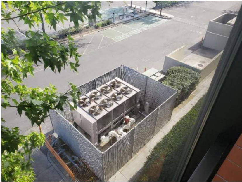
Photograph 9 – HVAC Equipment on the northeastern side of the building, from above.
