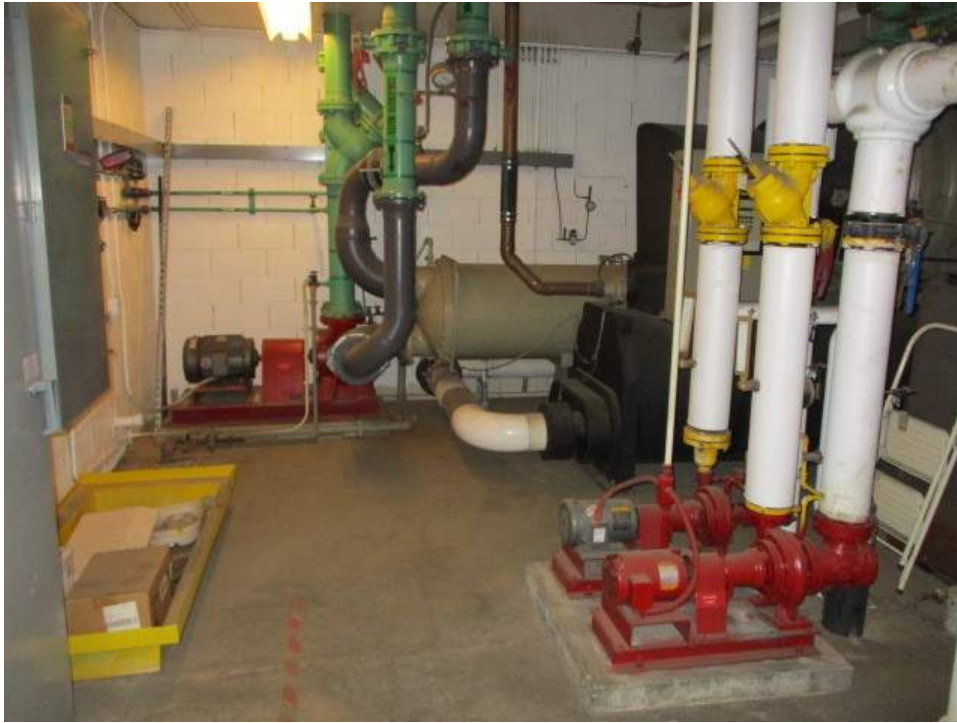
23. Water pump and HVAC equipment
