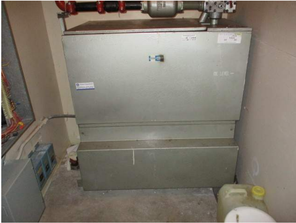
17. Hydraulic elevator unit
