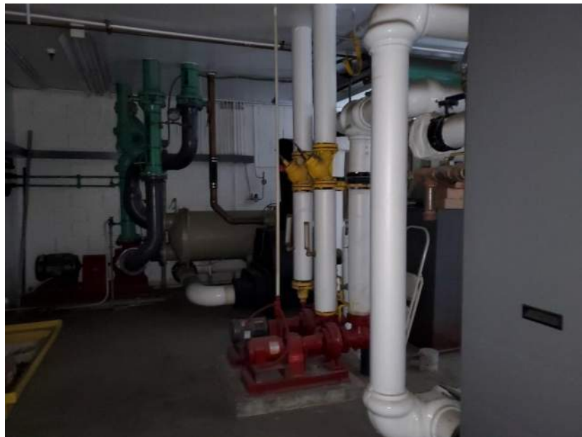
Photograph 28 – First floor mechanical room
