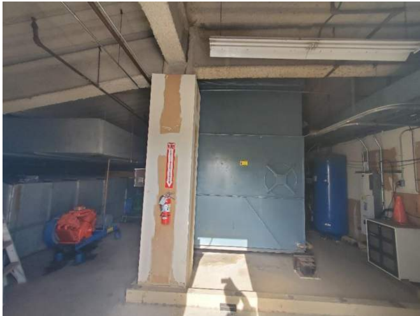
Photograph 18 – Mechanical room on the roof
