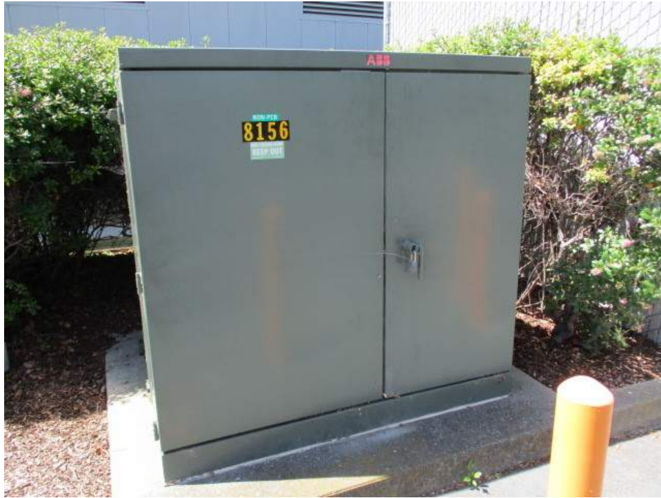
9. Pad-mounted transformer adjacent to the north of the building
