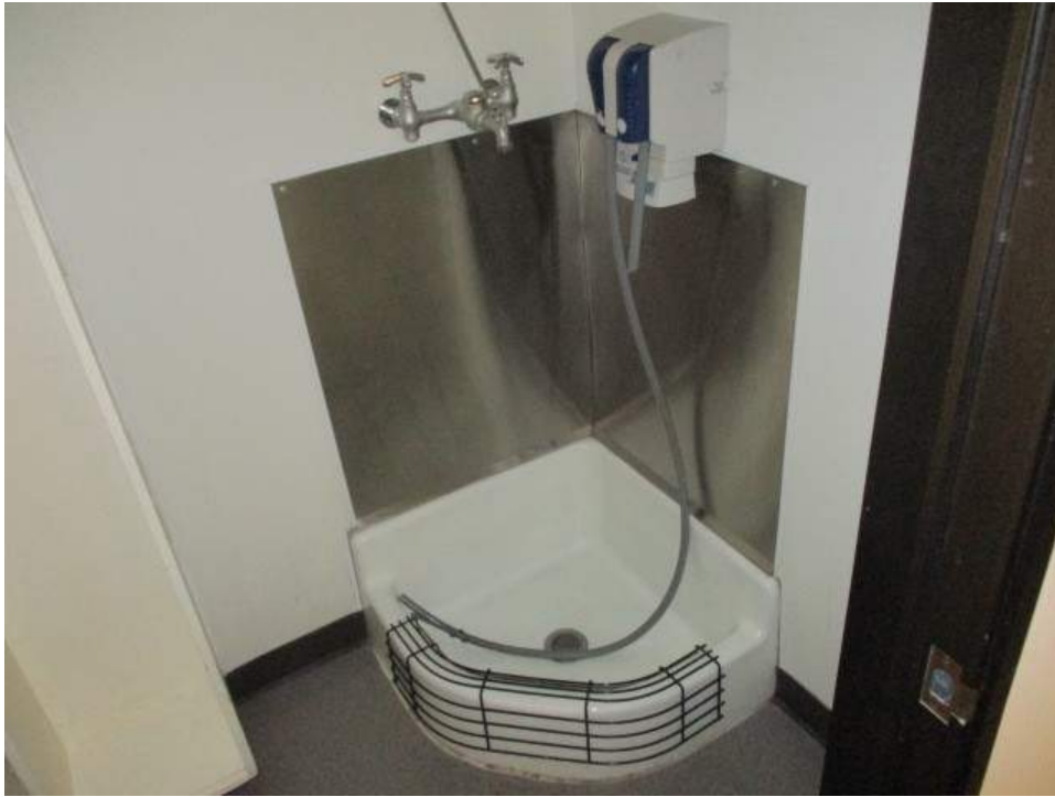
19. Floor sink in a janitorial closet
