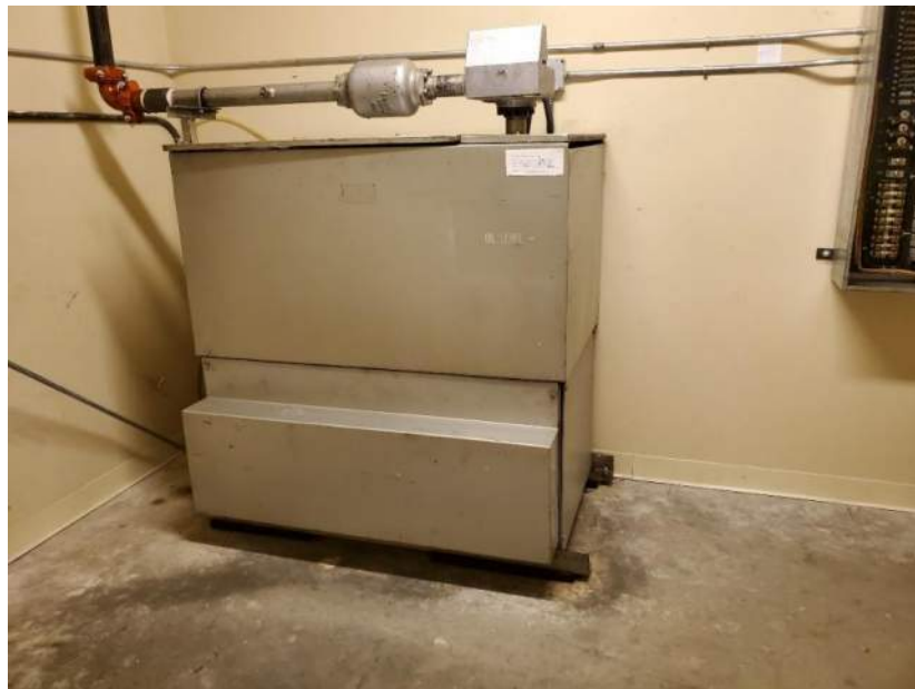
Photograph 20 – Hydraulic elevator unit in eastern elevator room
