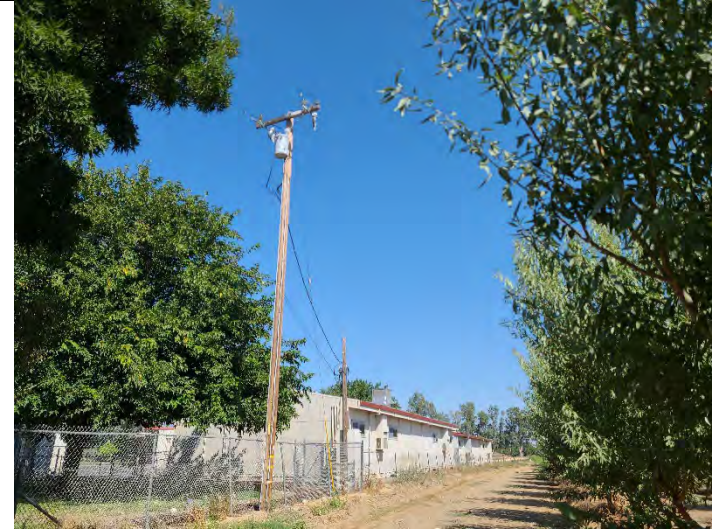
Photo No.4 – Electric Transformer, western boundary of Project Site.
