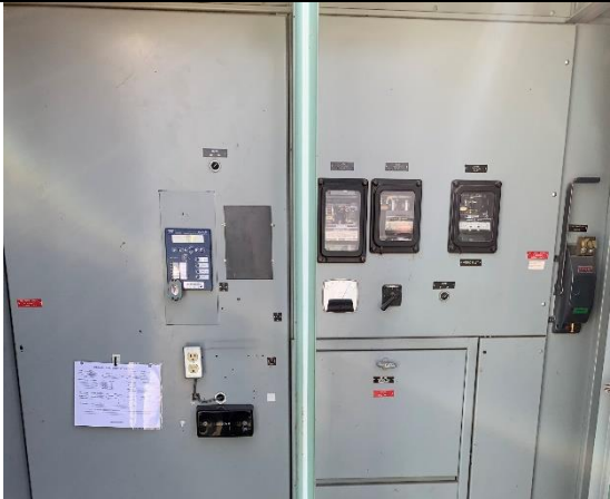
17-WAPA Power Meter (left side) (10-29-20)
