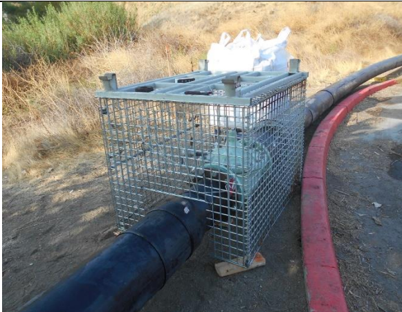
23-Cla Valve and Enclosure at Parking Lot (10-9-20)
