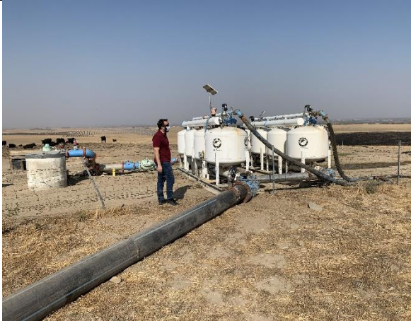
1-Filters in Operation (10-29-20)
