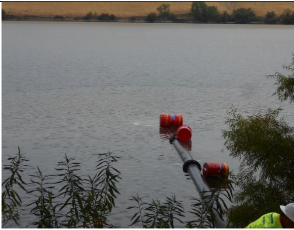
27-Discharge Pipe Floating (10-9-20)
