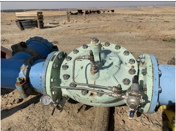
10-SLWD Furnished Valve at Filter Station (10-2930-20)
