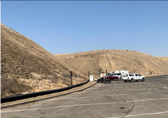
16-Pipe at Parking Lot (10-29-20)
