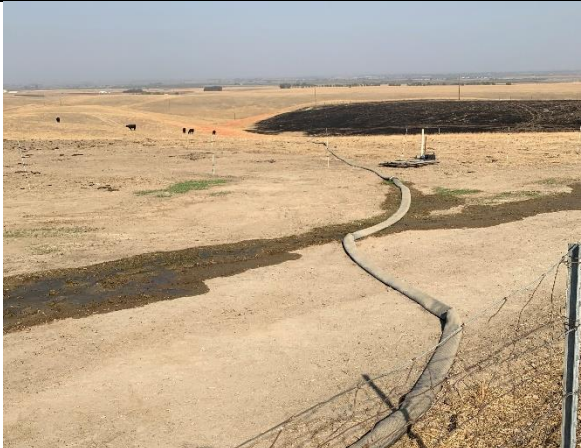
15-Layflat Pipe at Filters (10-29-20)
