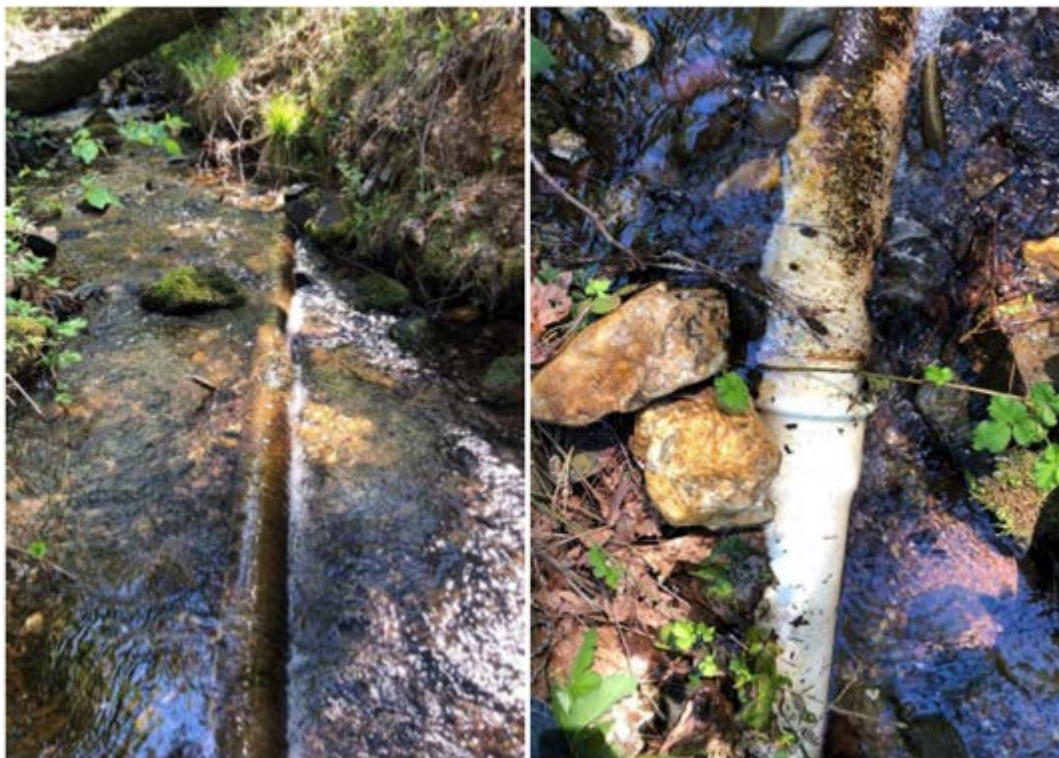
Existing Transmission Pipeline
