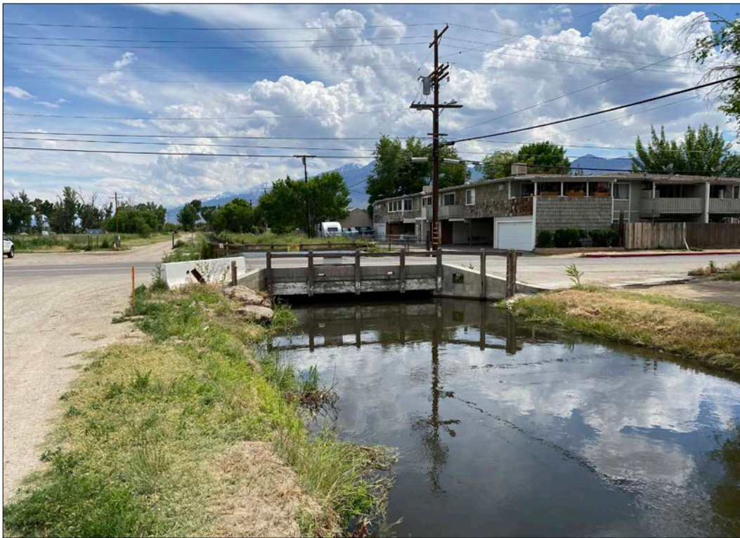
Photo 1. View of the of the East Line Street Bridge and Bishop Creek Canal looking south. Note that this is the location of the ordinary high water mark (OHWM)-1 cross section.
