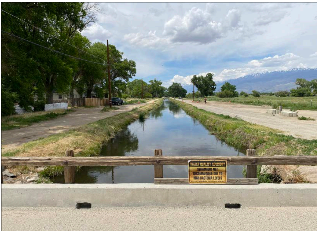
Photo 4. View of Bishop Creek Canal looking upstream to the north of the East Line Street Bridge.
