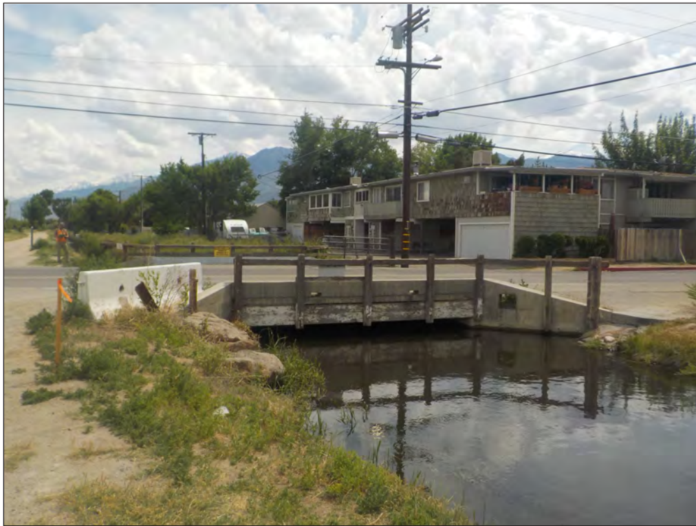
Photograph 7. View of bridge to be replaced from East side of Canal, taken on June 15, 2023 – facing Southwest.
