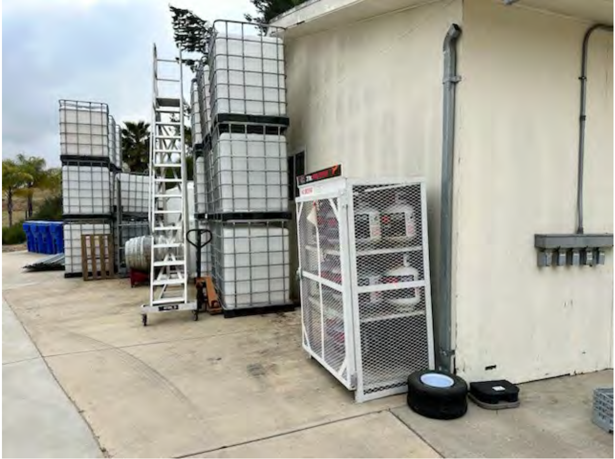
Propane tanks located on the north side of Wine Production Building.
