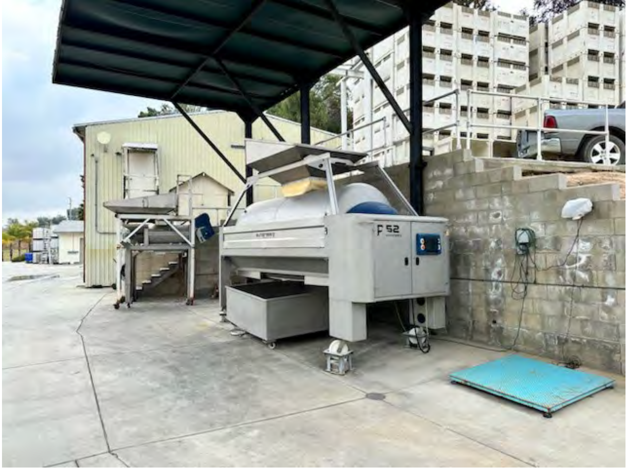
Equipment used in wine production, located immediately west of the Wine Production Building.
