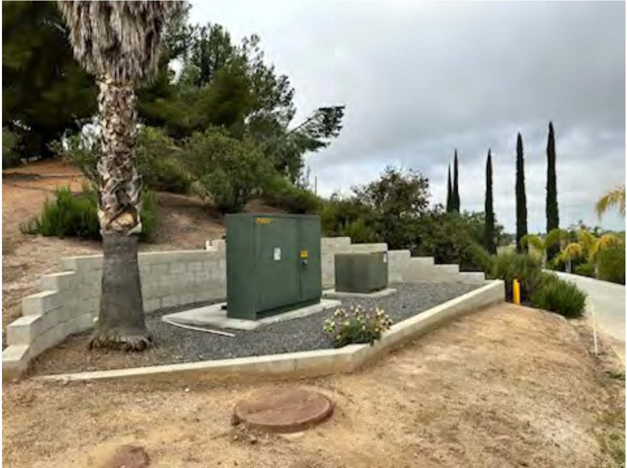
Pad mounted transformers located northwest of Wine Tasting Room.
