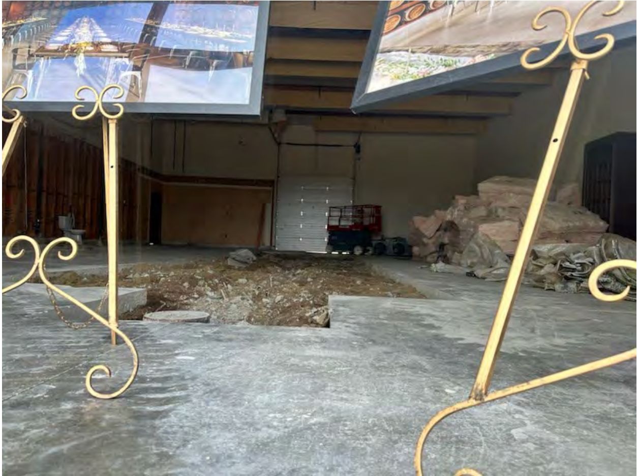
Interior of Barrel Room, under construction to be converted into a reception hall used by Wedgewood Weddings.
