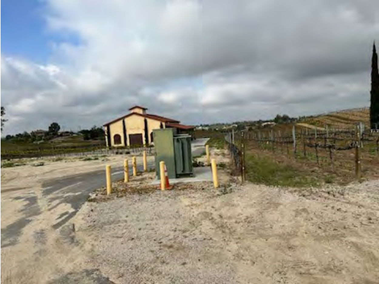
Pad mounted transformer located east of Barrel Room.
