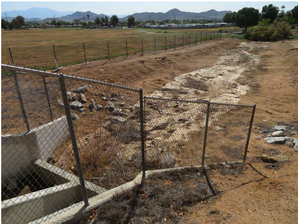
Photograph 8: View of the Hillman Street Storm Drain (HSSD) Channel in the southwest portion of the project site, facing southeast.
