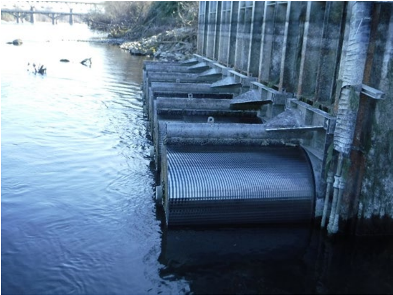
Figure 3. Existing PS1 Intake and Fish Screens
