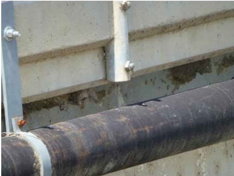
Photo #2 (below). Swallows were actively nesting on the Westwood Street bridge at the time of the April 17, 2018 field survey.
