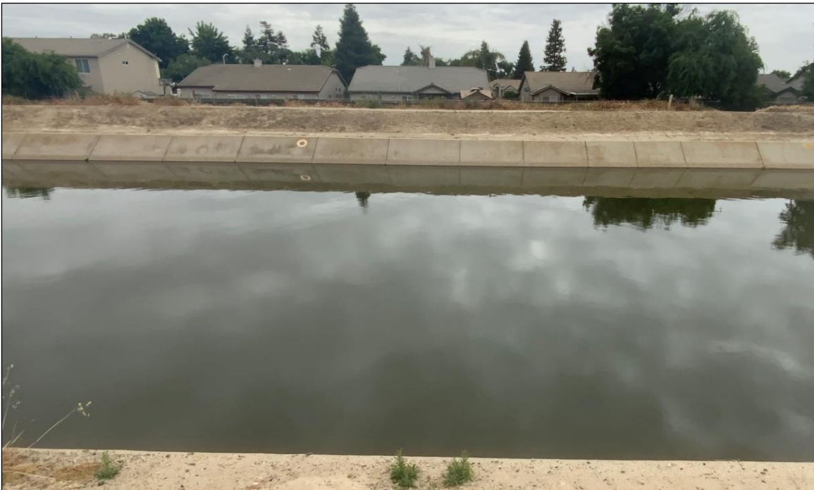
Figure 4-10 View of opposite (south) bank of Friant-Kern Canal with yellow circle indicating position of ladder on north bank, facing southeast.
