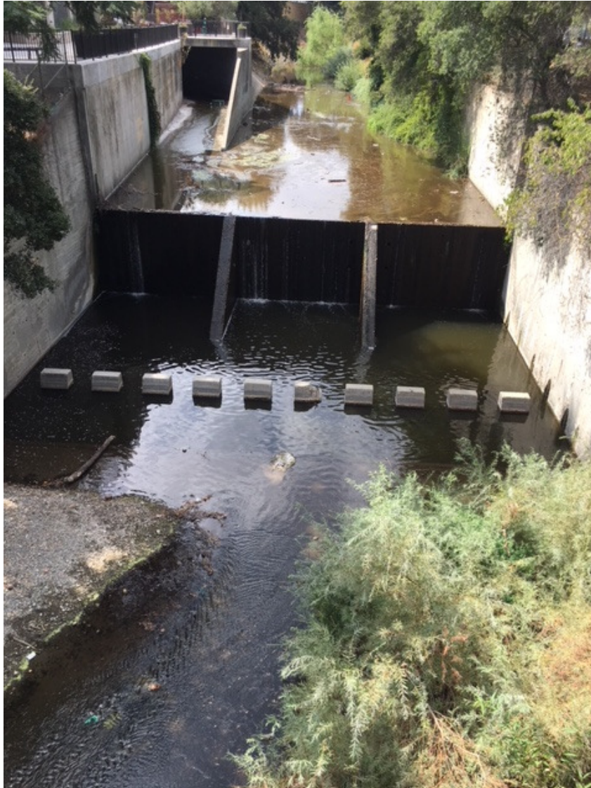
Photograph 1: View of Las Trampas Creek and confluence of Tice Creek (exiting culvert in top left of photograph) looking south from the South Main Street Bridge. Below the approximately 10-foot-high weir, two small gravel bars occur.
