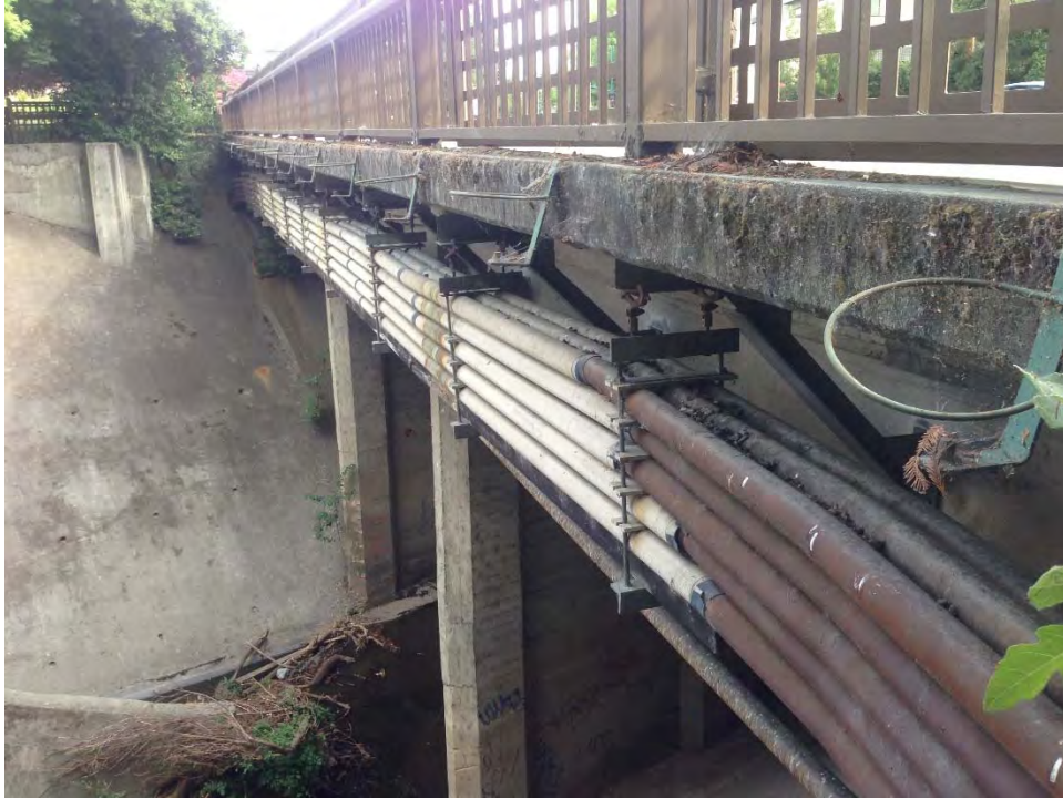
Photo 11. Closeup of utilities and transit-like pipe cover along east side of the bridge
