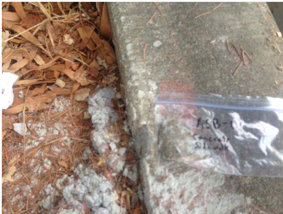
Photo 2. Sample ASB-01 taken from the concrete sidewalk along the western side of the bridge
