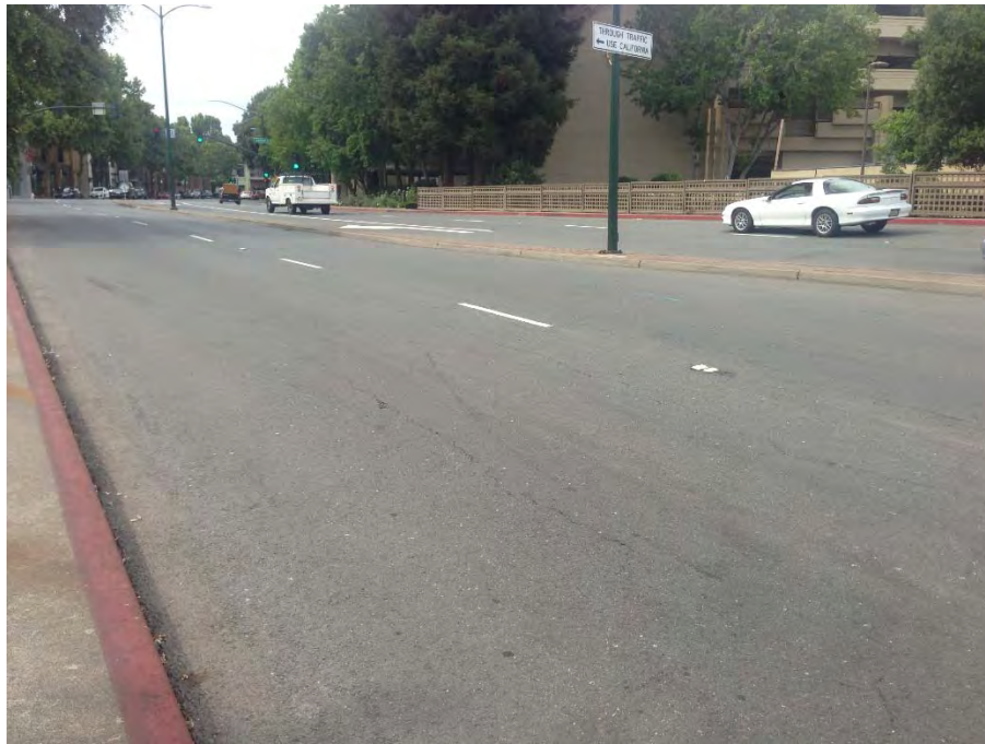
Photo 1. Looking NE towards parking structure on South Main St, Las Trampas Creek Bridge, overview of potential LBP and ACM sampling points
