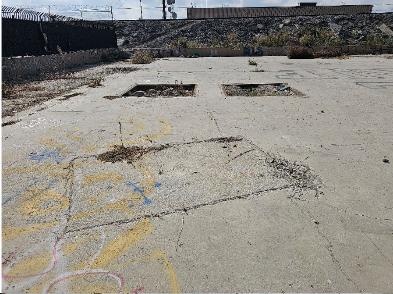
Photo 39: From center of structure pad, facing south, across dual access panels.
