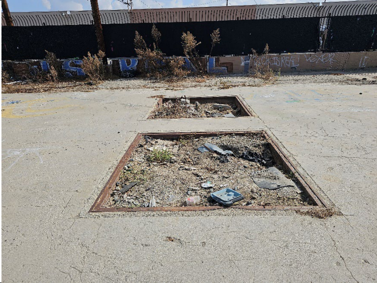
Photo 40: From structure pad, facing east, across dual access panels.
