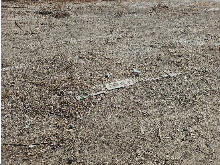
Photo 13: From western edge of property, plan view. Cinder block wall footings associated with previous auxiliary buildings extant in area on 1972 and 1988 historic aerial survey images.
