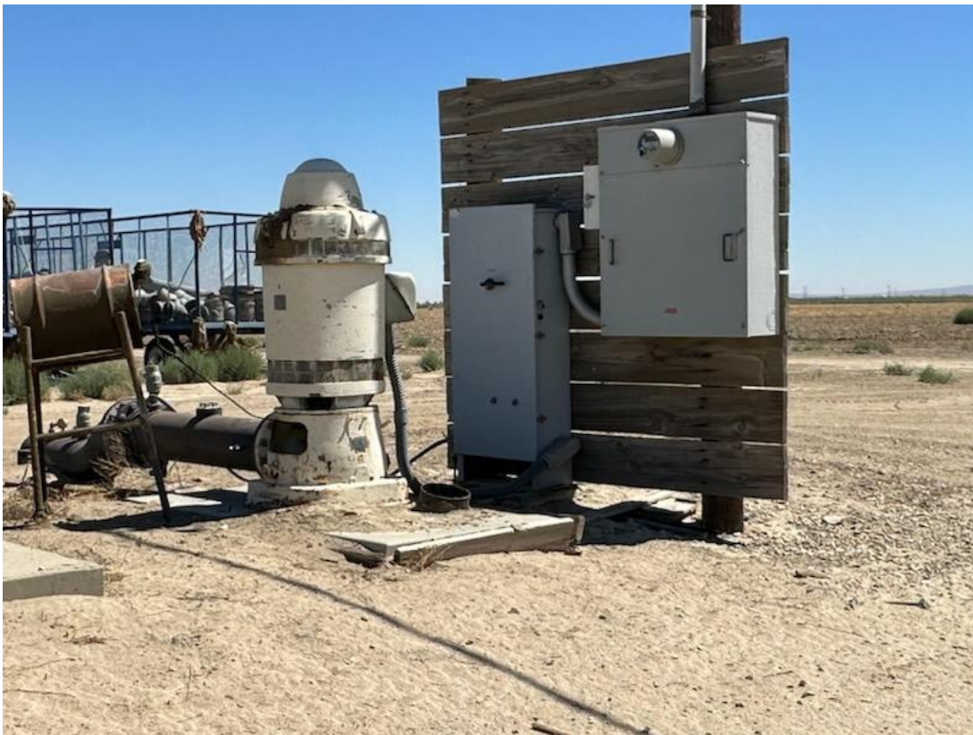
20. View of a groundwater pump located on the north-central portion of the Site.
