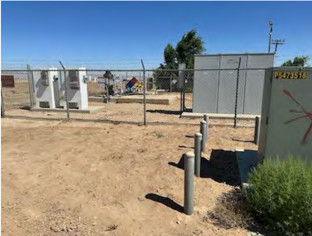
27. View of a groundwater pumping station at the southeast corner of the Site.
