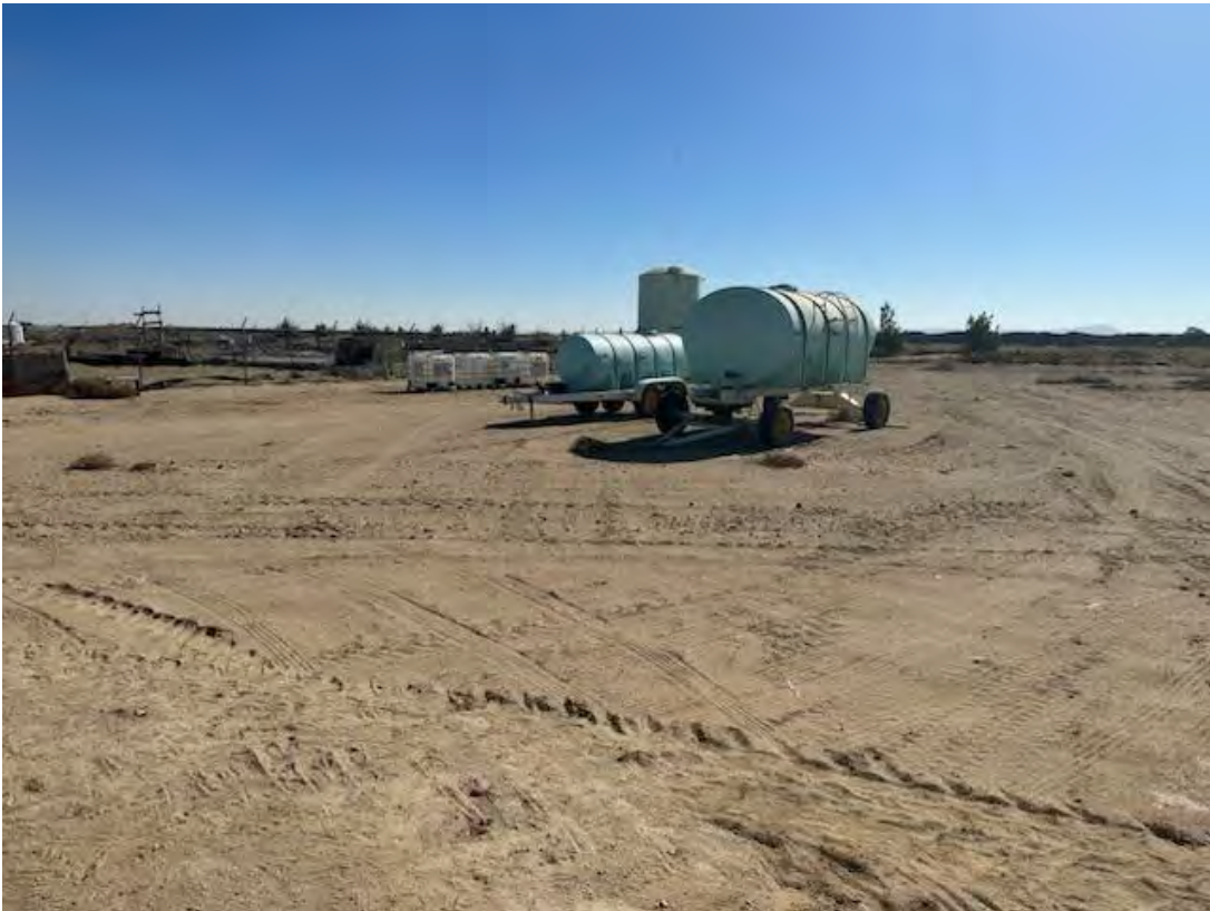
3. View looking at the work area near the middle of the Site.
