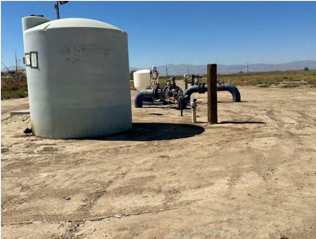
31. View of a pumping station on the eastern portion of the Site.
