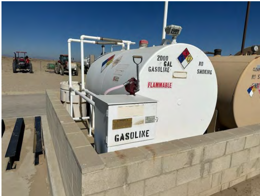
8. View looking at fuel station located in the work area near the middle of the Site.
