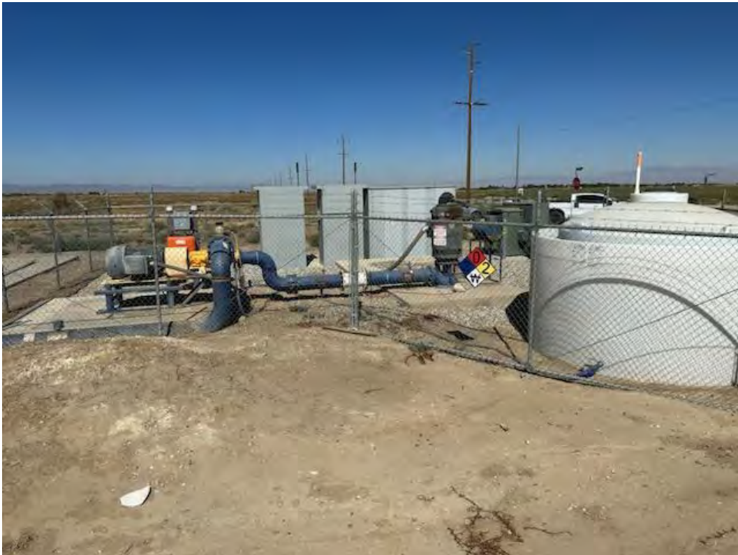
21. View looking at water pumping plant on the north-northwest corner of the Site.
