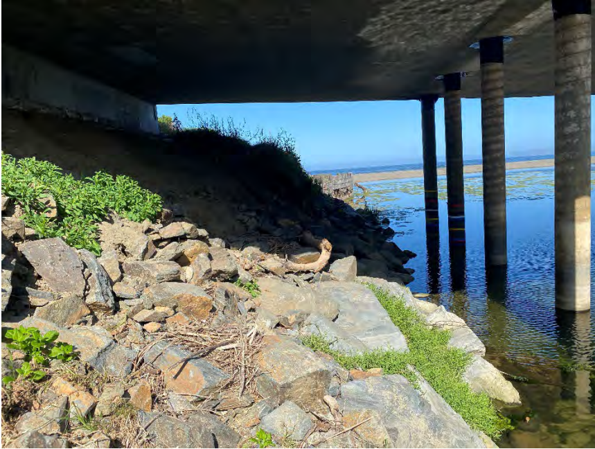
Photo 3. RSP on southern bank of Toro Creek under SB bridge looking west.
