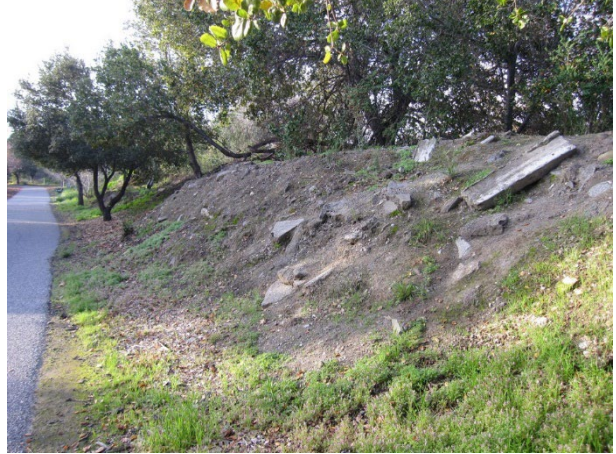
Photograph 6. Debris between trail and creek.
