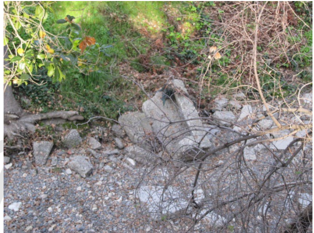
Photograph 8. Concrete debris in Saratoga Creek channel.
