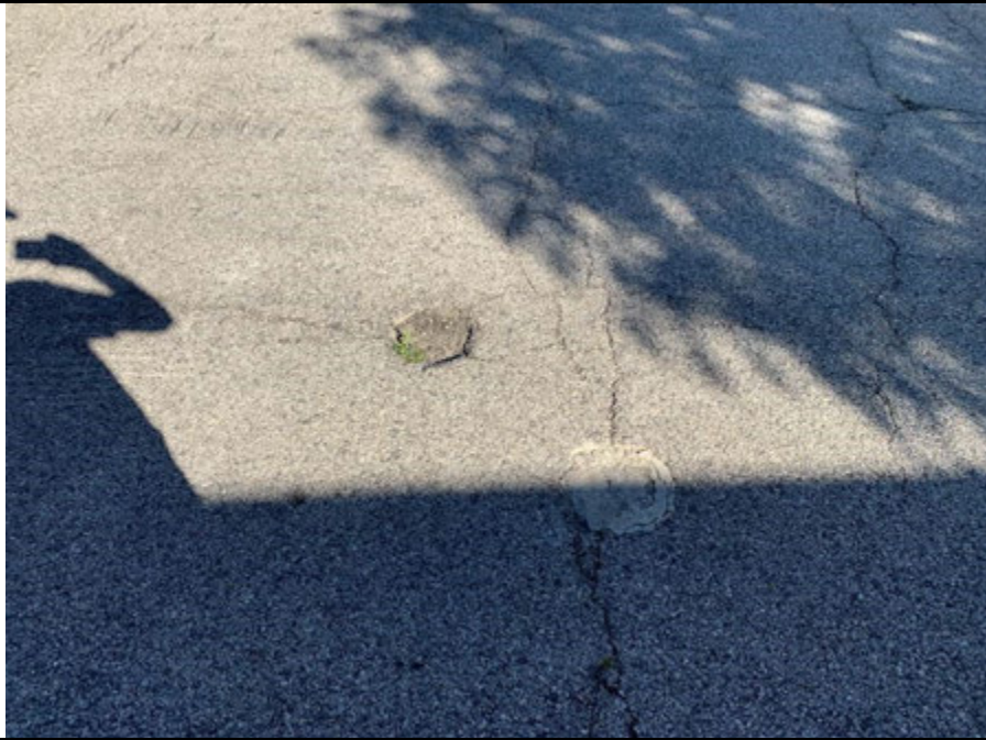
Photo 9: View of an 8-inch asphalt patch and a 10-inch concrete patch in the parking lot north of the building on Site.
