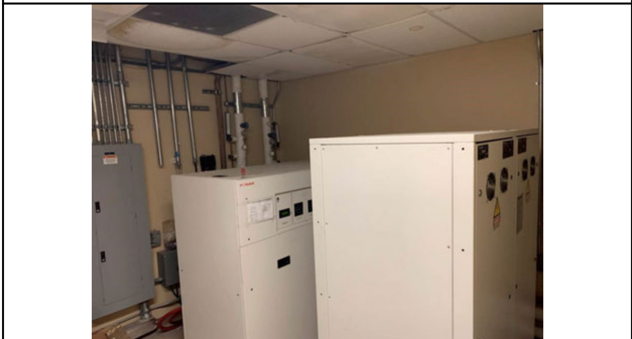
Photo 8: View of electrical room housing units related to MRI machines.
