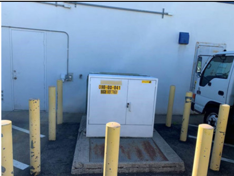
Photo 10: View of a pad-mounted transformer on the north side of the building (western end).
