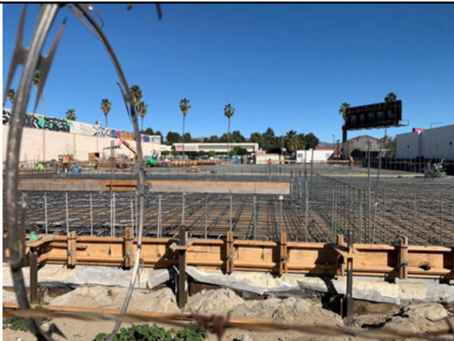
Photo 14: View of new construction on the north adjoining property, looking north (20112 Sherman Way).
