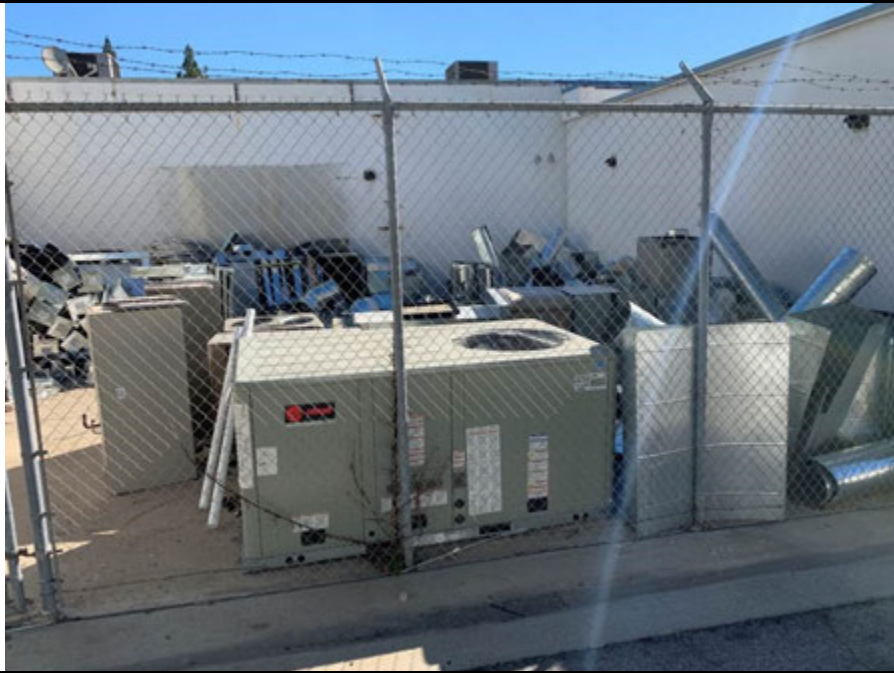
Photo 11: View of several HVAC units on the west side of the building.
