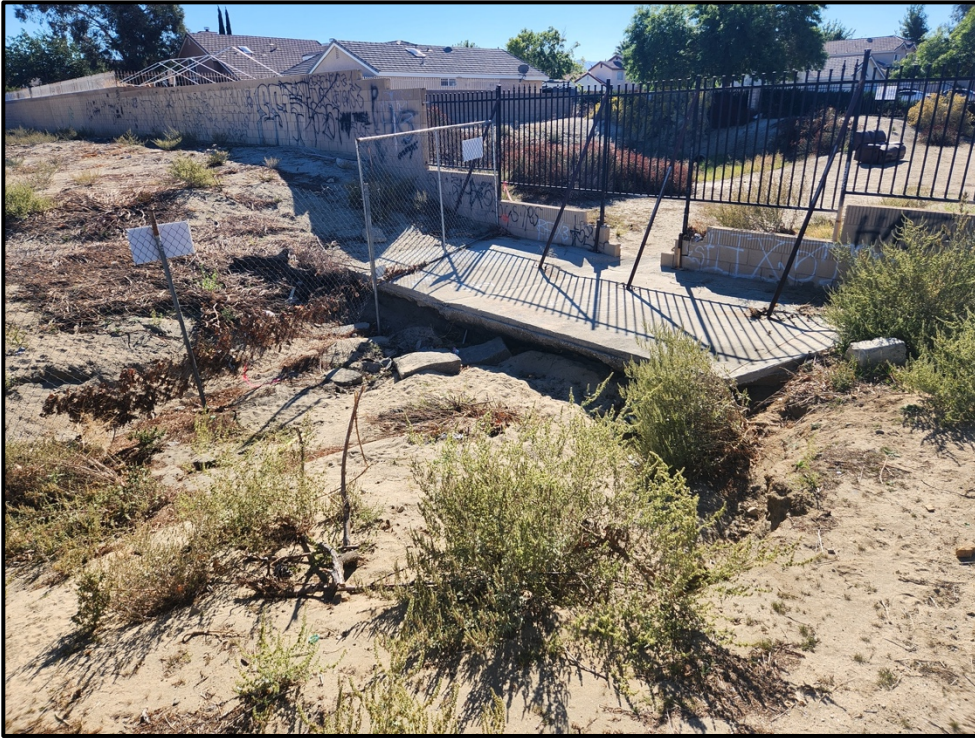
Plate 3.2–3: View of the modern culvert and earthen ditch located in the southeast corner of the project, facing southeast.
