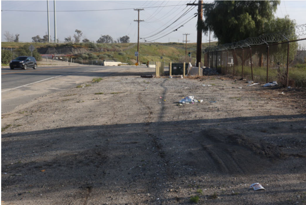
Figure 8. Photograph (March 7, 2023) of the parking Alternative site #3 on the south side of Agua Mansa Road (view looking east toward the Rialto Channel crossing (background). Roadside conditions are with a well compacted gravel base.
