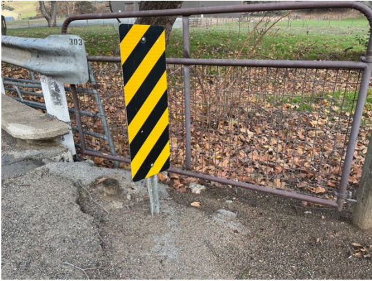
View of wooden post stump behind Type P object marker on northern side of Bridge 303. December 20, 2022. Facing northwest.
