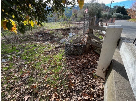
View of embankment on the east side of Bridge 302. December 20, 2022. Facing south.
