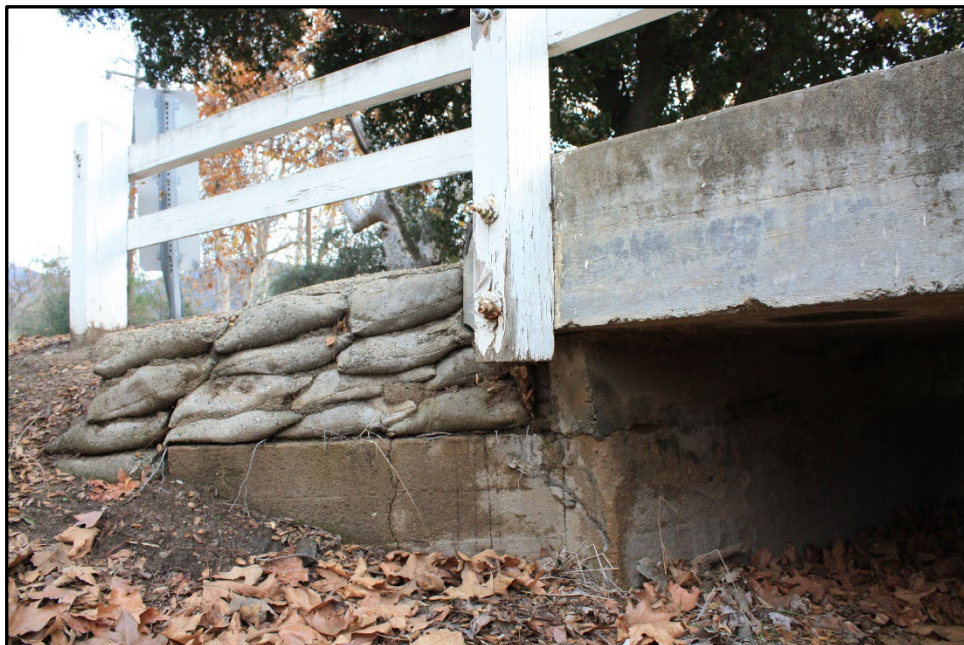
Photograph 3: Bridge 302, showing the east side abutment where slump concrete sits atop the original board formed concrete; camera facing east; December 19, 2022.
