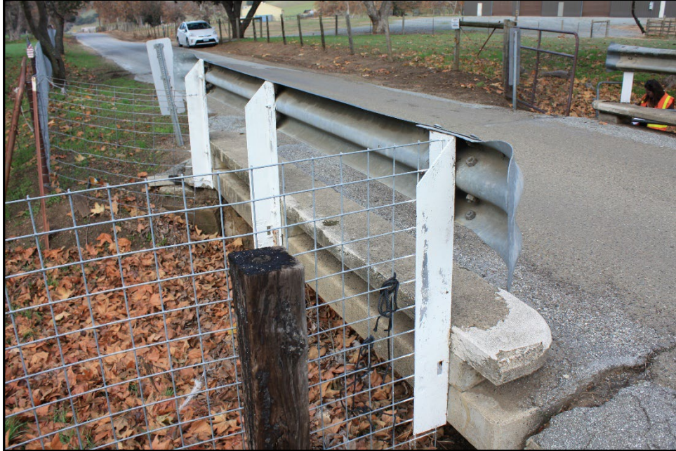
Photograph 8: Bridge 303, showing its south side wheel guard and how the guard rail blots into the deck; camera facing northwest; December 19, 2022.
