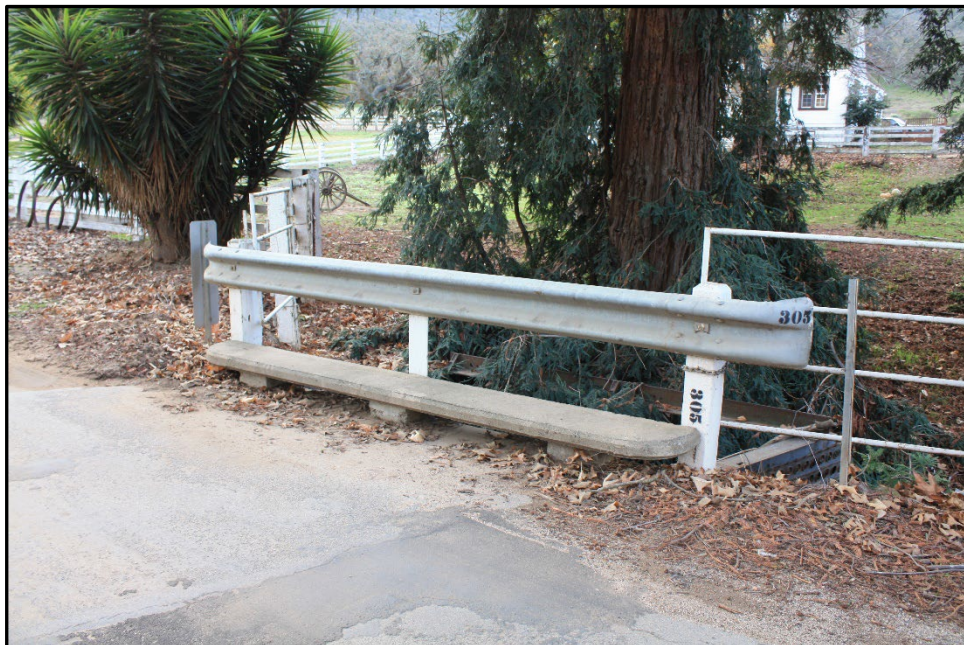
Photograph 15: Bridge 305, showing the wheel guard and guard rail; camera facing southeast; December 19, 2022.
