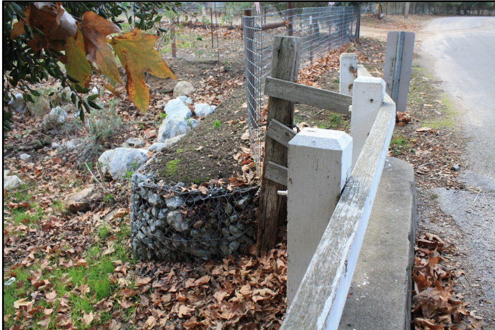
Photograph 4: Bridge 302, showing the rock filled wire basket supporting its southwestern wing wall; camera facing south; December 19, 2022.
