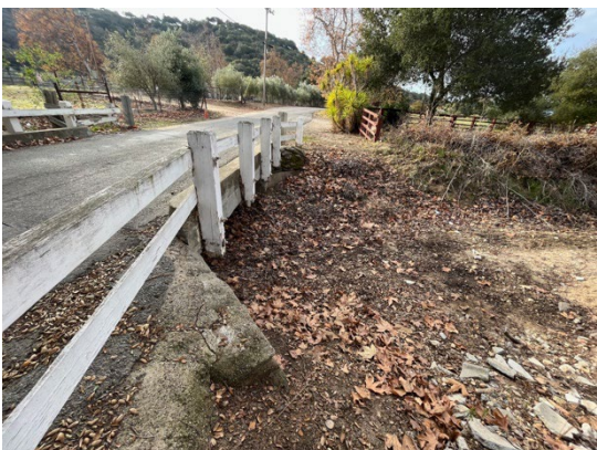
View of west side of Bridge 302 over the Chualar Creek drywash. December 20, 2022. Facing south.
