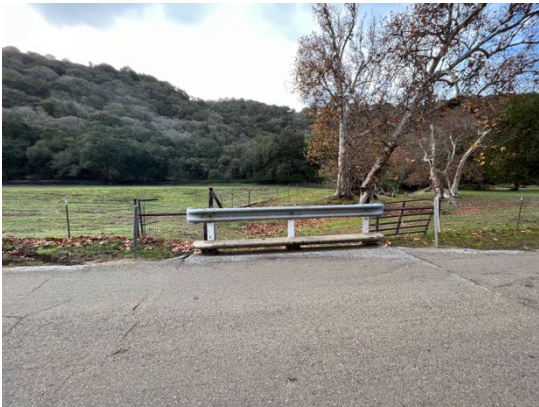
Guardrail on southern side of Bridge 303. December 20, 2022. Facing south.
