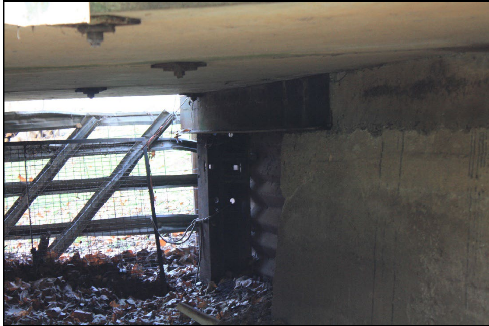
Photograph 10: Bridge 304, showing where the northern edge of the east abutment has been extended; camera facing south; December 19, 2022.
