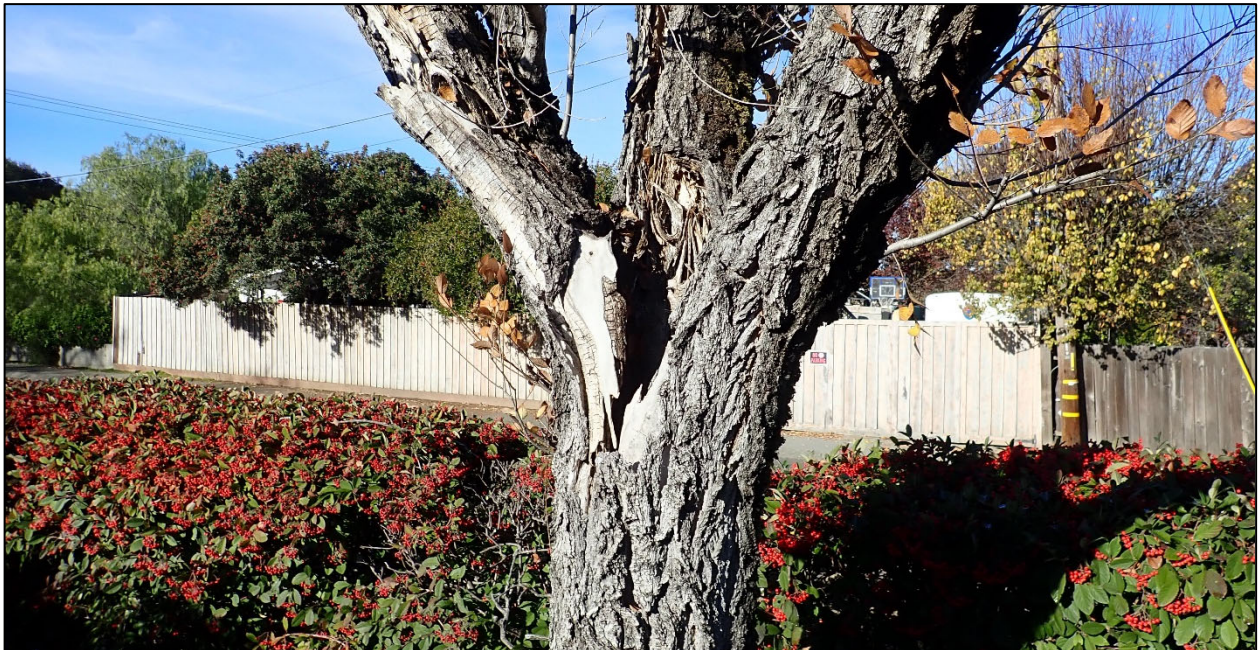
Photograph 2. Photograph depicting Siberian elm tree #582 at Site 1. The tree in poor condition, exhibiting a large internal cavity affecting the tree's health, structure, and condition.
