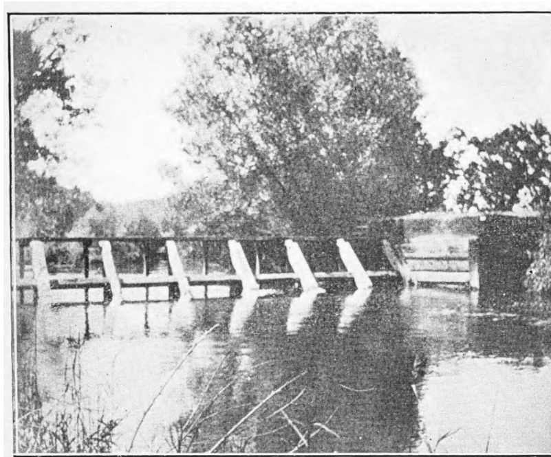
Figure 3. Photograph of the Murphy Slough headgate shared by the Turner and Riverdale ditches. Source: Harry Barnes, Plate X in Bulletin No. 7: Use of Water from Kings River, California. California State Printing Office, Sacramento, 1920.
