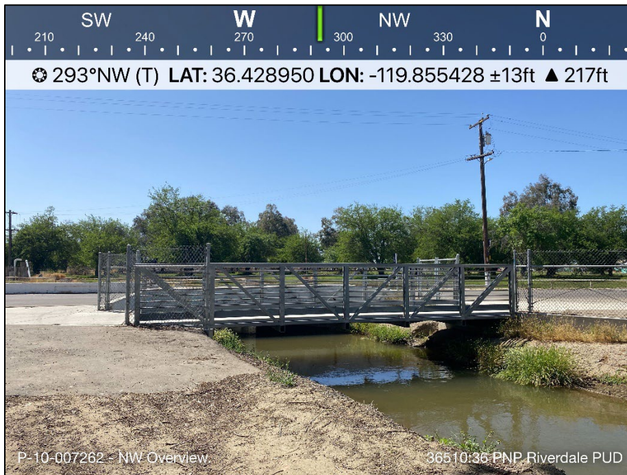
Figure 12. Overview of bridge on S. Feland Avenue crossing the Burrell Ditch (P-10-007262), looking northwest.
