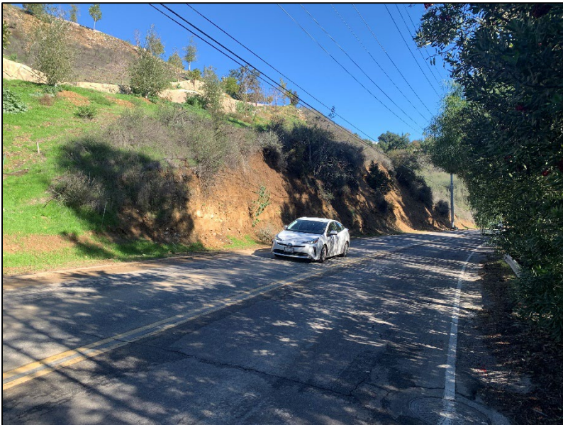
c. Slope to be stabilized with steel netting, north of Parksouth Street
