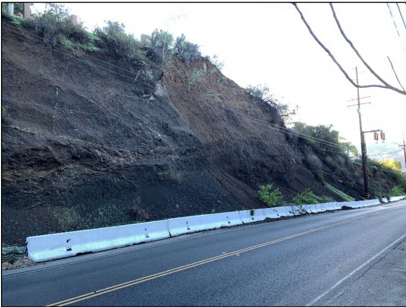
a. Slope to be stabilized with pinned shotcrete near Turtle Creek Road
