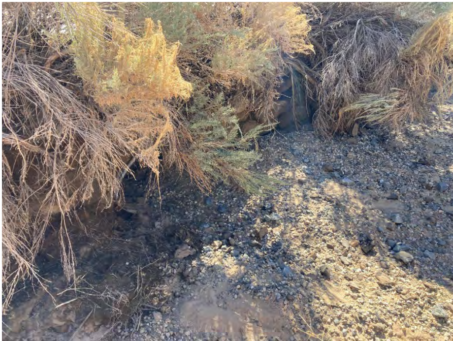
Photo 4. View of drainage pipe on the eastern portion of the Project site, which connects to the existing natural earthen channel across 10 th Street East; facing east. Taken September 2022.
