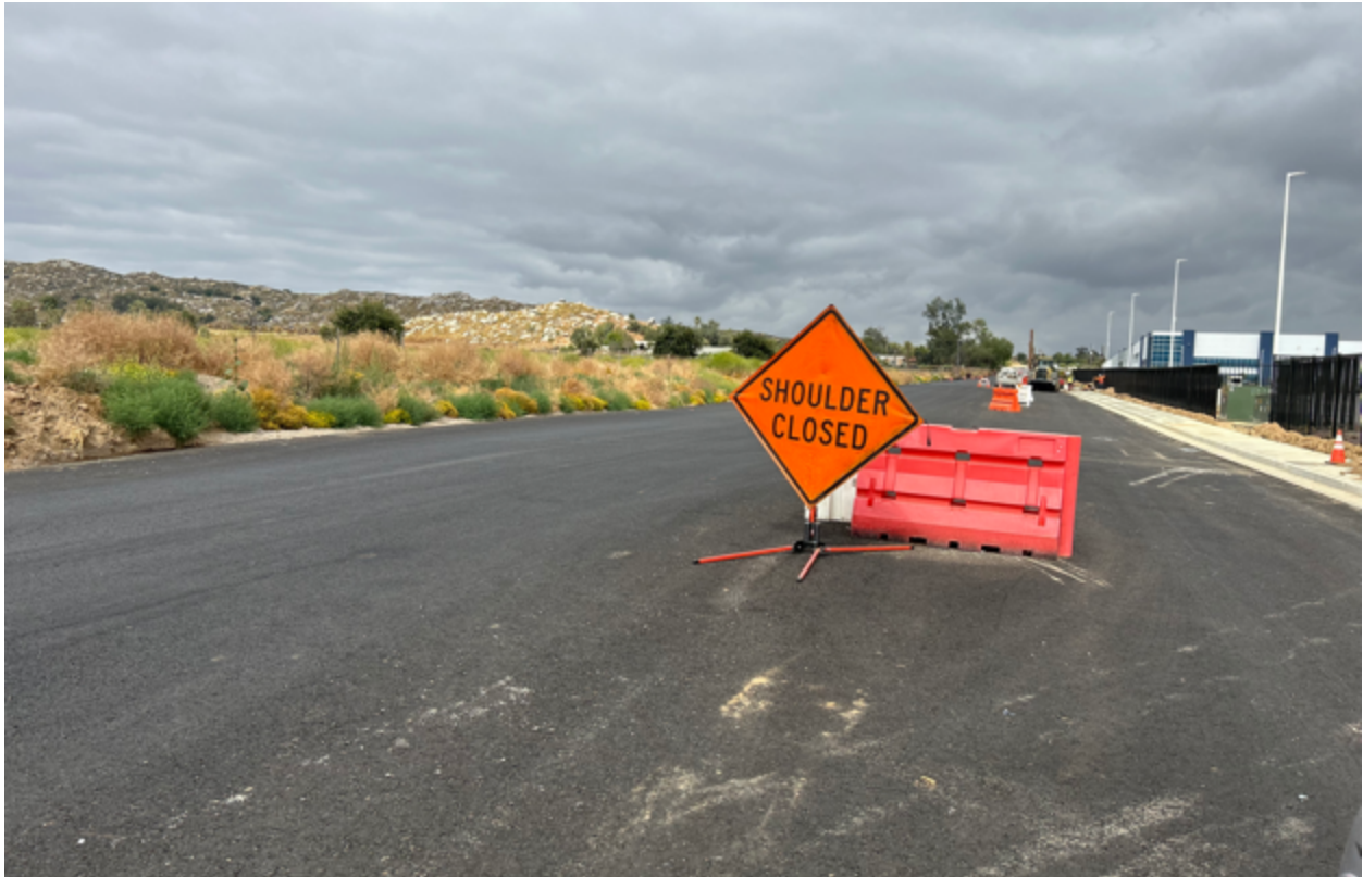
Photo 14. Corner of Harvill Avenue and Placentia Street. Looking west down Placentia Street.
