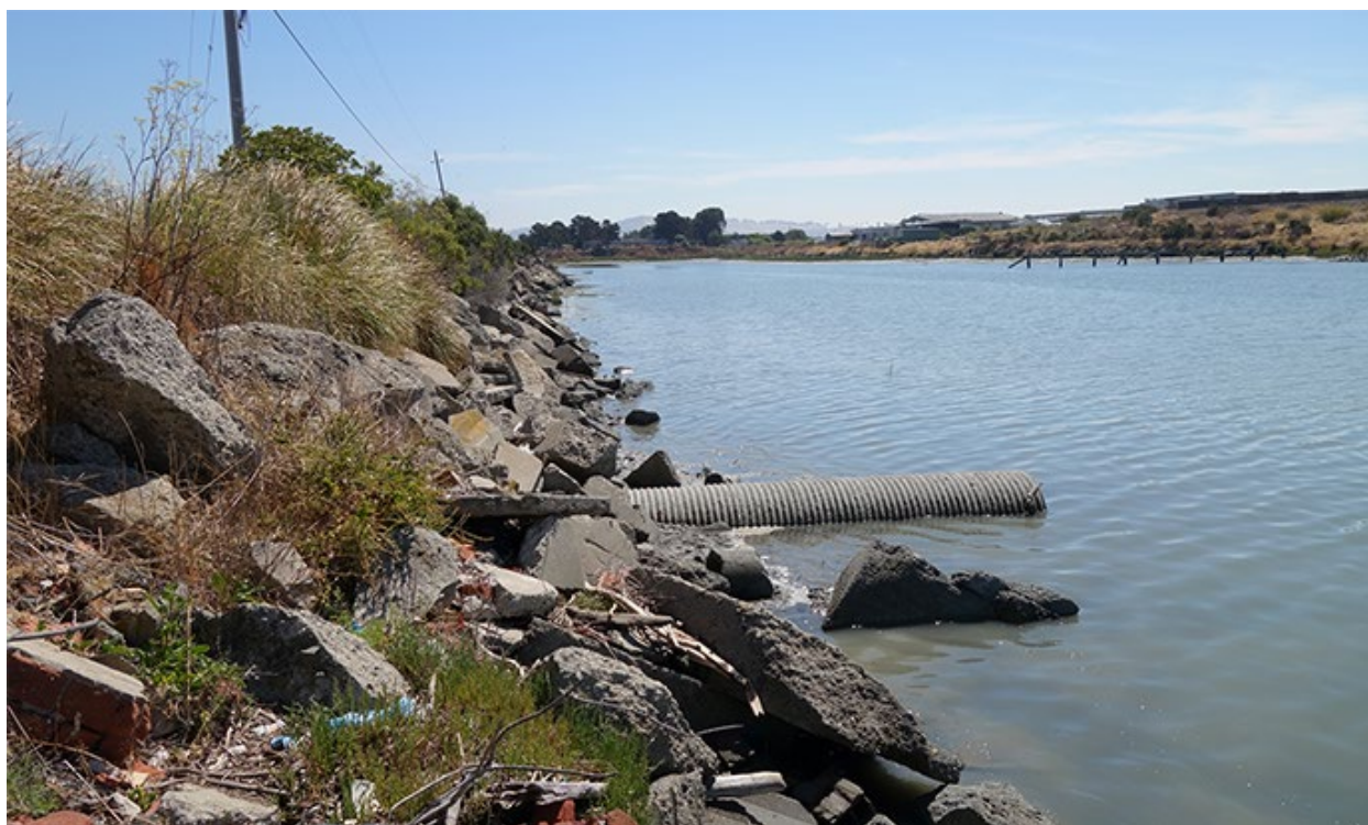
Figure 2.8. Existing conditions – east-facing view of the outfall to the tidal slough south of the existing basin
