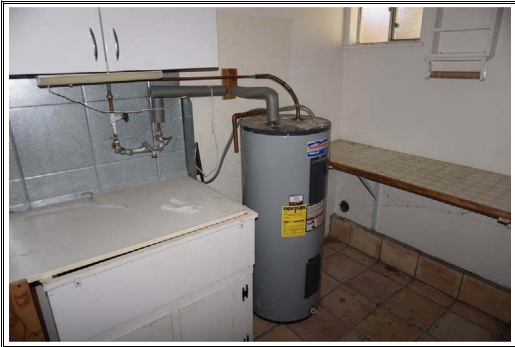
Photograph Number 42: View of electric hot water heater within barn.
