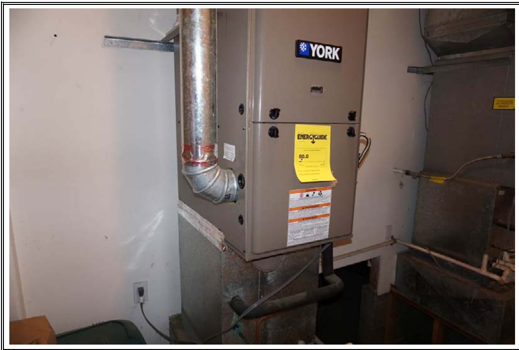
Photograph Number 36: View of natural gas furnace within dwelling.
