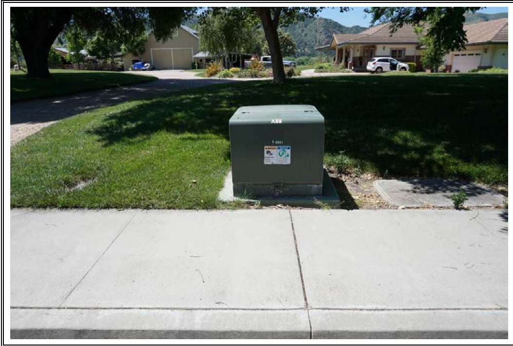
Photograph Number 5: View of on-site pad-mounted transformer along Dairyland Road, facing southwest.
