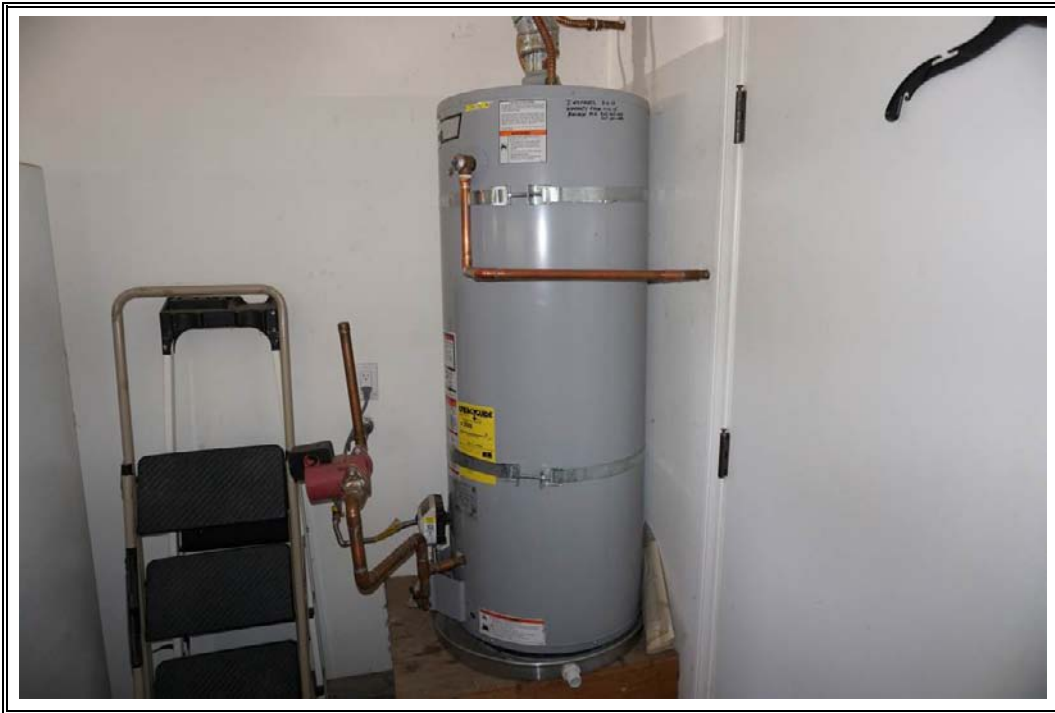
Photograph Number 35: View of natural gas hot water heater within dwelling.
