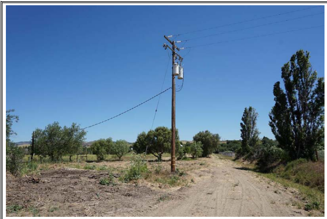
Photograph Number 26: View of two pole-mounted transformers on southern corner of subject property, facing northeast.
