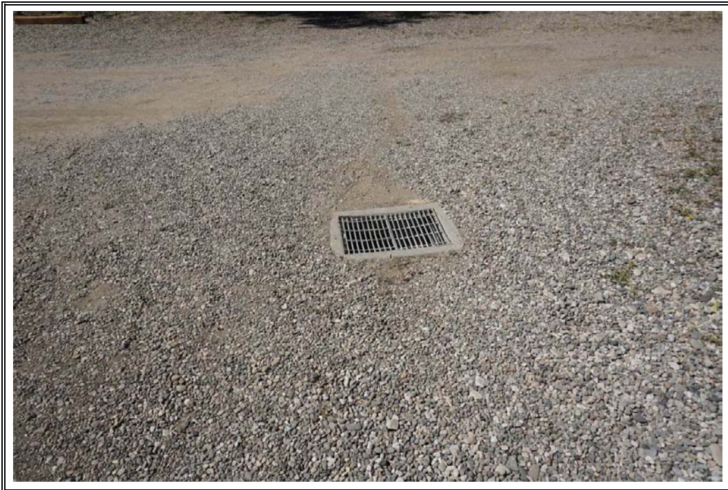
Photograph Number 17: View of one of several storm water drains located throughout the subject property.
