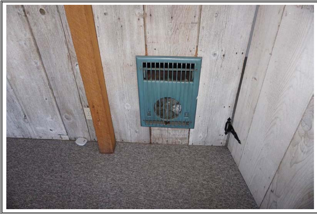
Photograph Number 45: View of electric heater within studio loft apartment.
