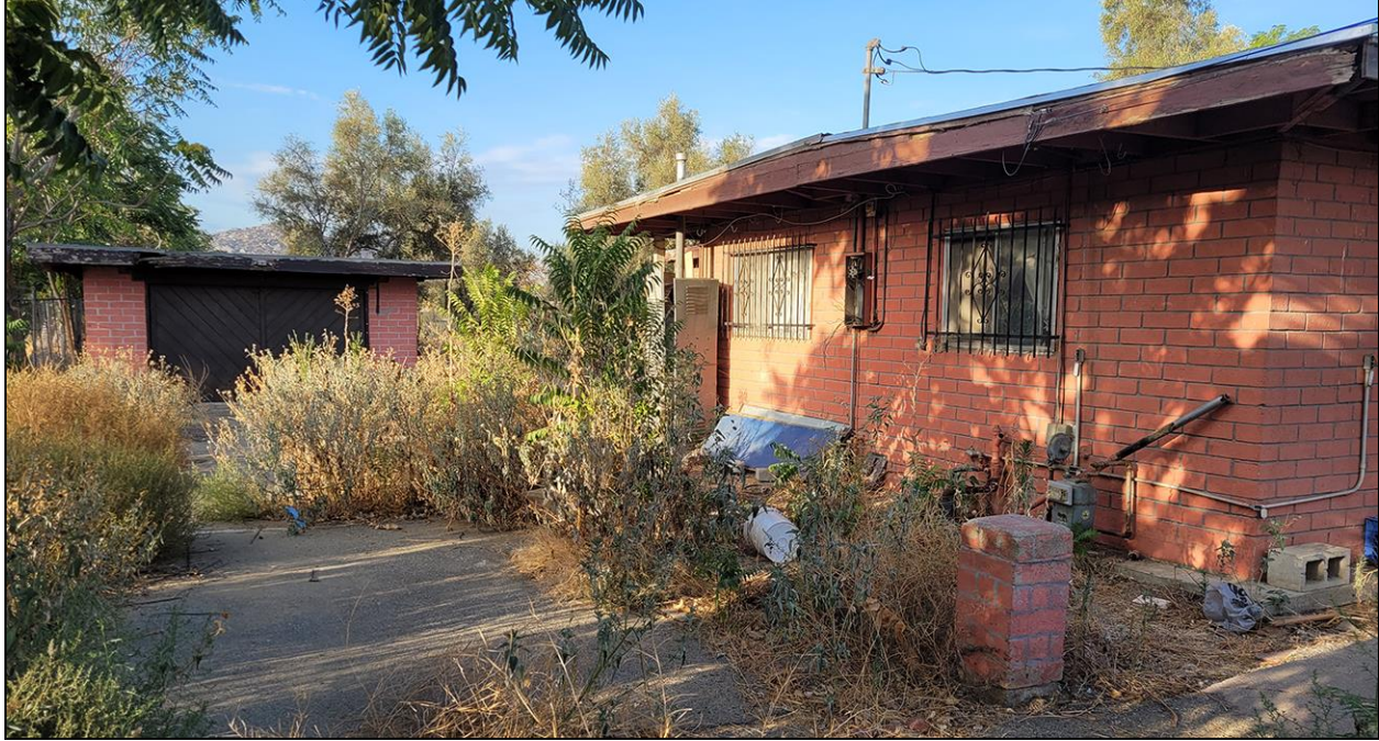
East side of the main residence and north side of the converted garage (view to the south)
