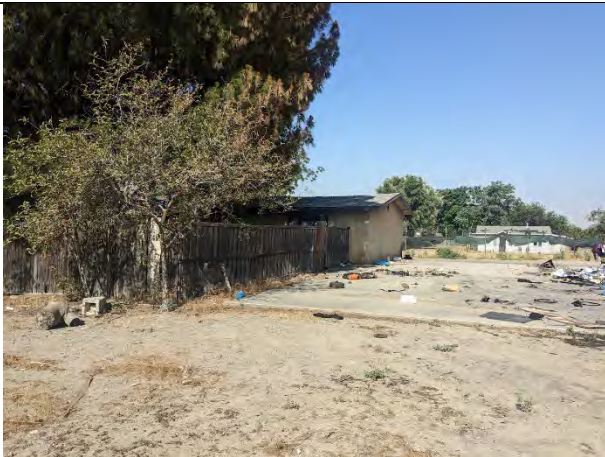
Photo 9. Looking west toward exposed foundation at 16264 Slover Ave.
