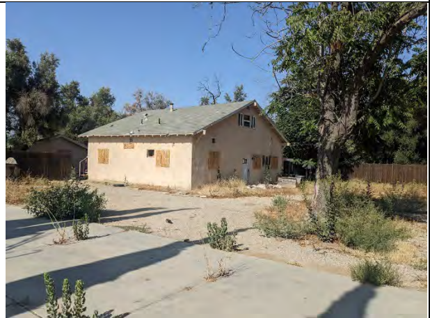
Photo 10. Looking southwest toward boarded up residence at 16283 Boyle Ave. Note the presence of openings that may allow for bats or other animals to enter the structure.
