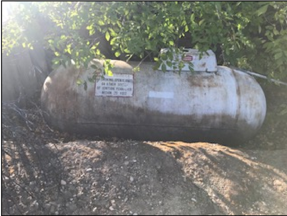
IMG_0907 - 500 gallon above ground propane tank inside the entrance to the residential plot.
