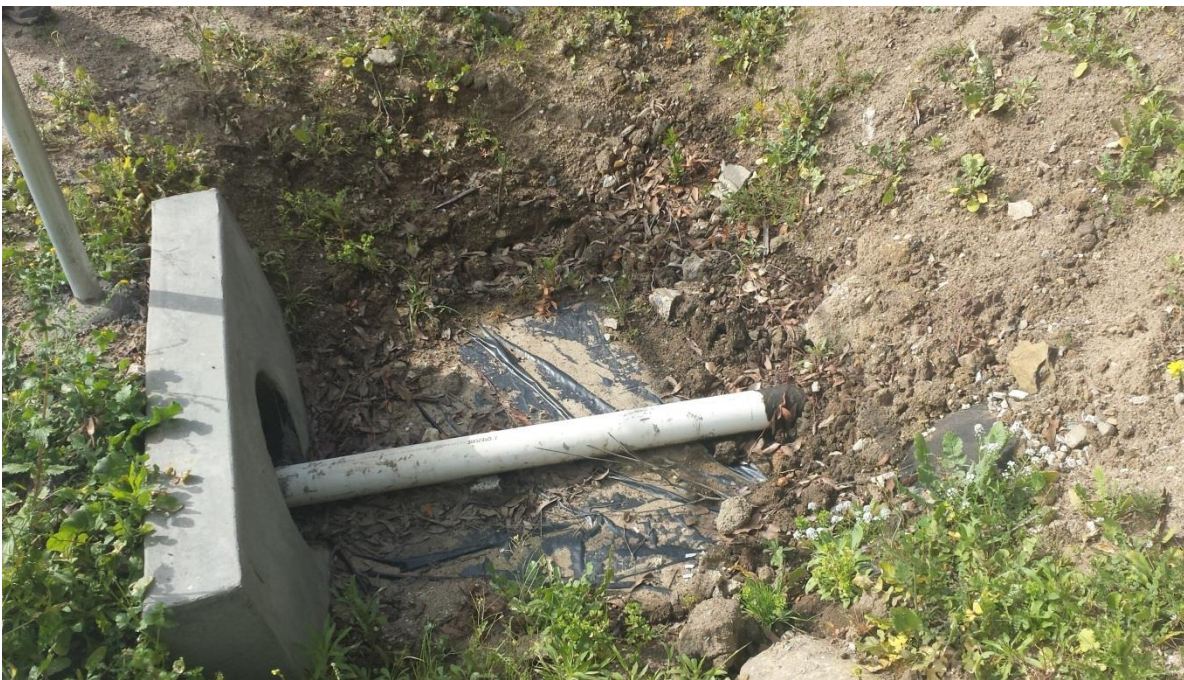
Photograph 14. The beginning of the drainage that crosses the northern portion of the project site. This location is off the project site, located at the northwestern corner of the dirt drive leading up to the two residences. The pipe appears to carry water into the drainage from off-property.
