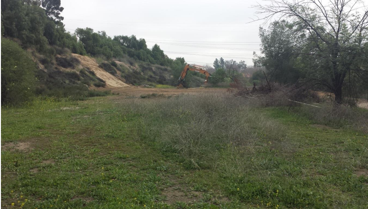
Photograph 3. View looking east across the southern portion of the site with ruderal vegetation, California buckwheat scrub on the slope, and a cleared area with heavy earth-moving equipment present. At the time of the survey, Ararat Home had not purchased the project site; therefore, the earthwork depicted in this photo was presumably conducted by the property owners at that time.
