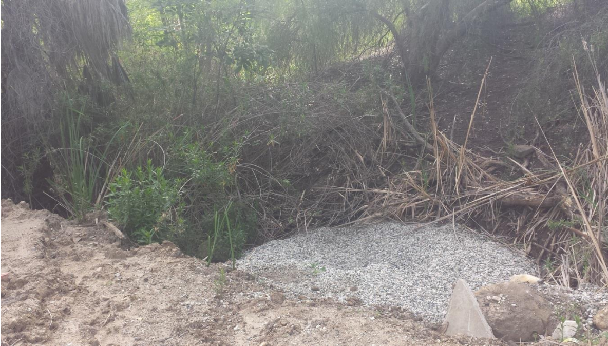
Photograph 13. View looking southeast from the northwestern corner of the project site at drainage that crosses the northern portion of the project site, including a culvert (lower right corner) and gravel.
