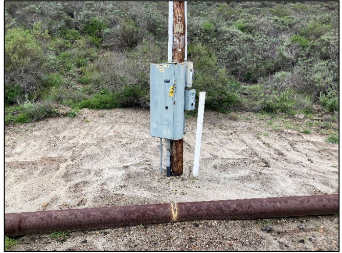
Photograph 14. View of pole location 3 (white stake), adjacent to an existing pole and within the bare ground and ruderal footprint of the existing pole.
